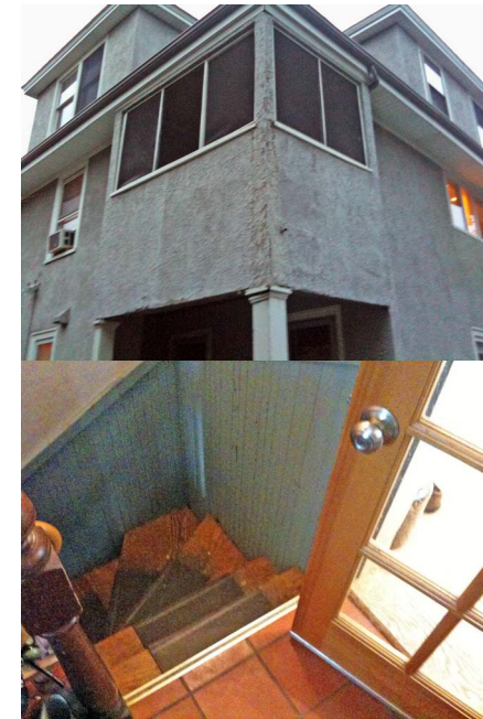
2010 - dilapidated rear entry and dangerous winder stair.
