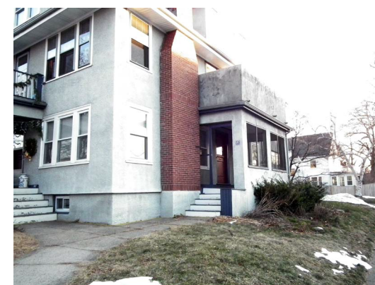
2012 - Eyesore of Spruce St. porch had rotted wood foundation.
