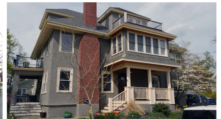
In 2012 we removed and redesigned the Spruce St. porch with an attractive second story and third floor open deck on a new foundation.
