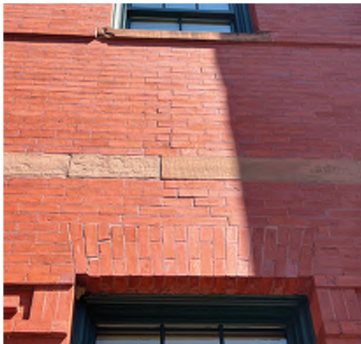
Image A-22: Slipping jack arch and step cracking at ground floor windows at south elevation Note widened joint at arch.
