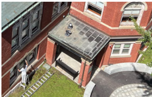
Image B-06: Flat seam copper roof over east portico. Evidence of ponding present around spotlights.
