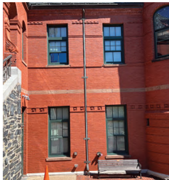
Image A-20: View of inset copper gutters at the south elevation. Copper gutters typically drain into cast iron boots.
