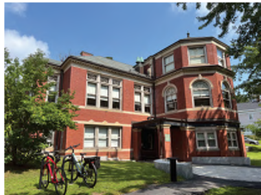
Image B-29: View of the southeast corner of the building showing various types of original and new windows
