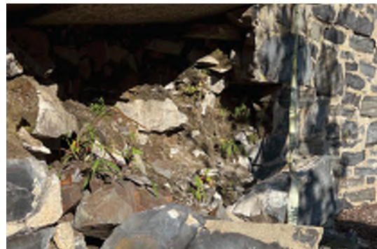
Image A-53: Dry-laid stone retaining wall backfilled with soil, no other structural support present.
