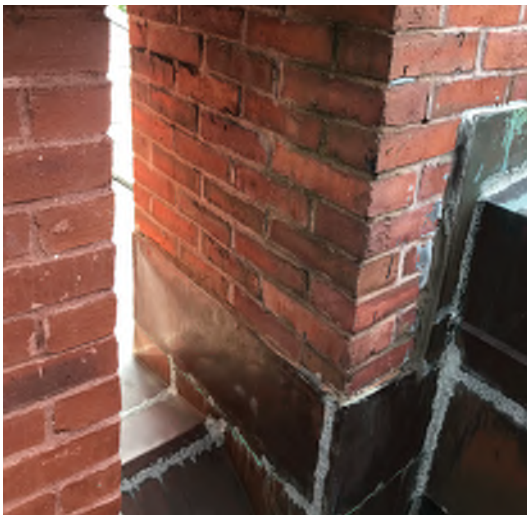
Image B-14: Poorly detailed copper counterflashing detail at chimney. No visible clips and new sealant joints required.
