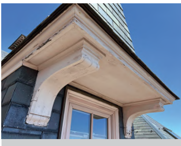
Image C-31: Most paint on the dormers require light scraping and a new coat.
