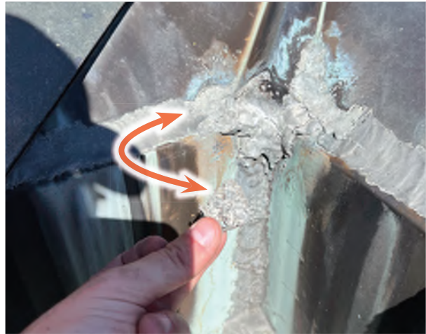
Image C-23: Large chunks of broken-off solder are indicative of unskilled application.
