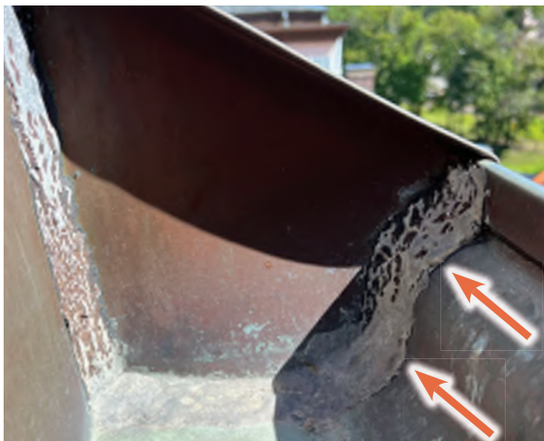
Image C-21: Hairline cracks at solder joints are a site for water to infiltrate the wood cornice below.
