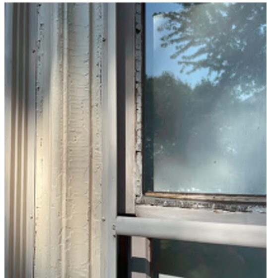
Image B-30: Close up of original window showing cracked glazing putty, aluminum storm window, and wood trim.
