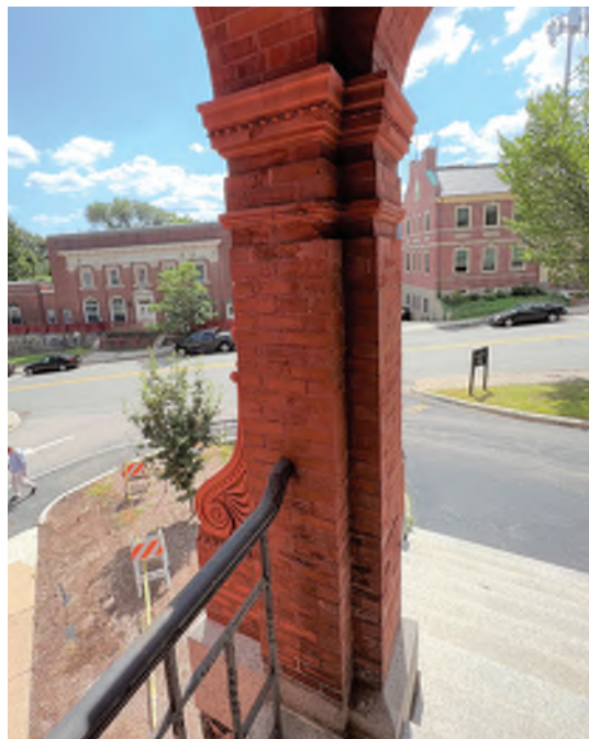
Image A-26: Deteriorated and spalling brick masonry at the interior of support column at south portico.
