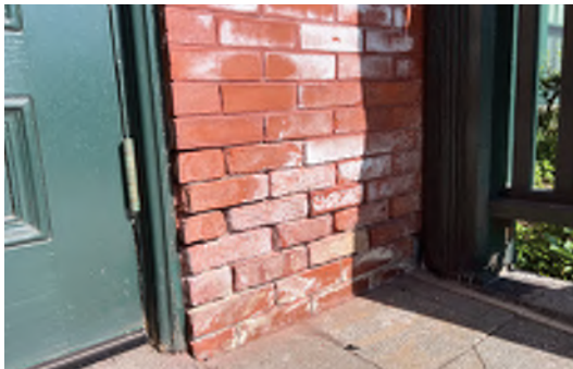
Image A-28: Deterioration and efflorescence at base of east entry vestibule causing by rising damp and de-icing salts.
