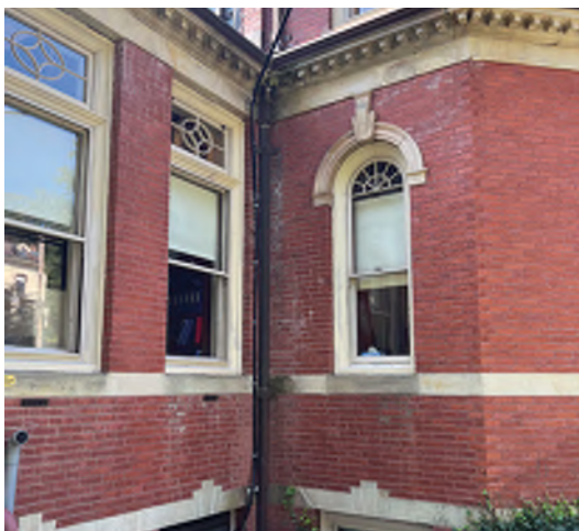
Image B-21: Severe brick masonry and mortar deterioration caused by ineffective copper gutters and downspouts.
