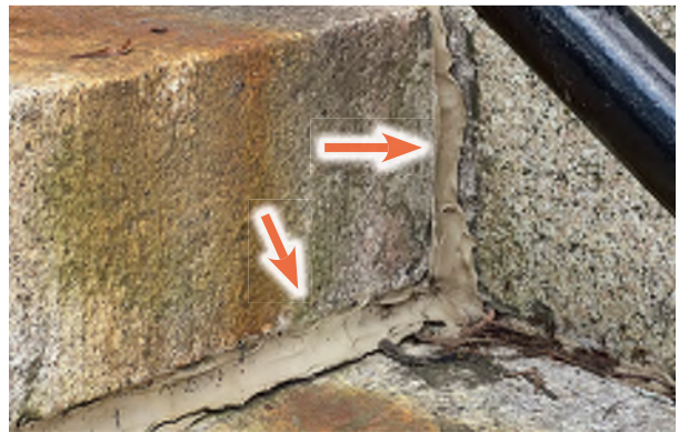
Image C-56: The slow shifting of granite treads are filled with sealants, wider and wider with each application.
