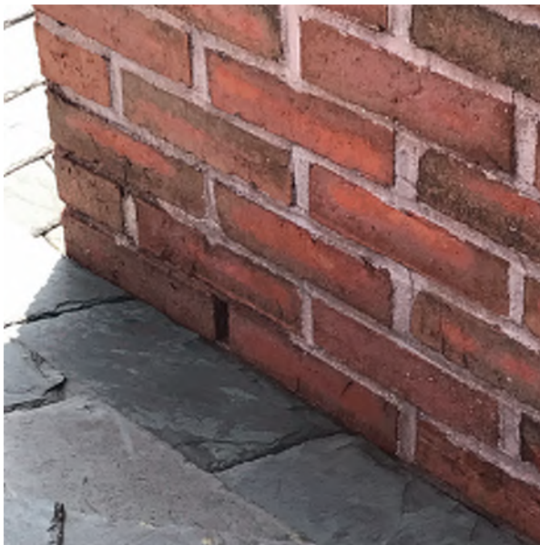
Image B-11: Open mortar joint at the rear face of the south chimney caused by water and snow accumulation off of the elevator override.
