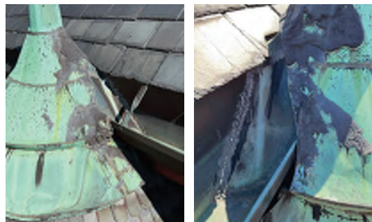
Image A-13: Heavy mastic and other patching to prevent water infiltration at questionable gutter intersection.
