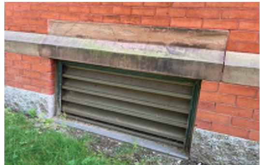
Image A-32: Staining, scaling, and open joints at brownstone watertable typical across the building.
