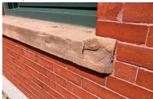
Image A-49: Deterioration of brownstone sills across the Belmont Town Hall.
