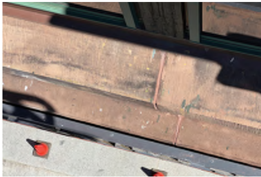
Image A-51: Sky-facing joints at large brownstone sills are susceptible to water infiltration and deterioration.
