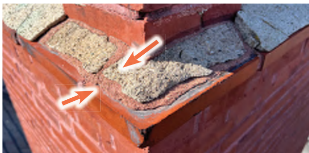
Image C-45: An earlier red-tinted mortar wash and the chimney should be re-applied.
