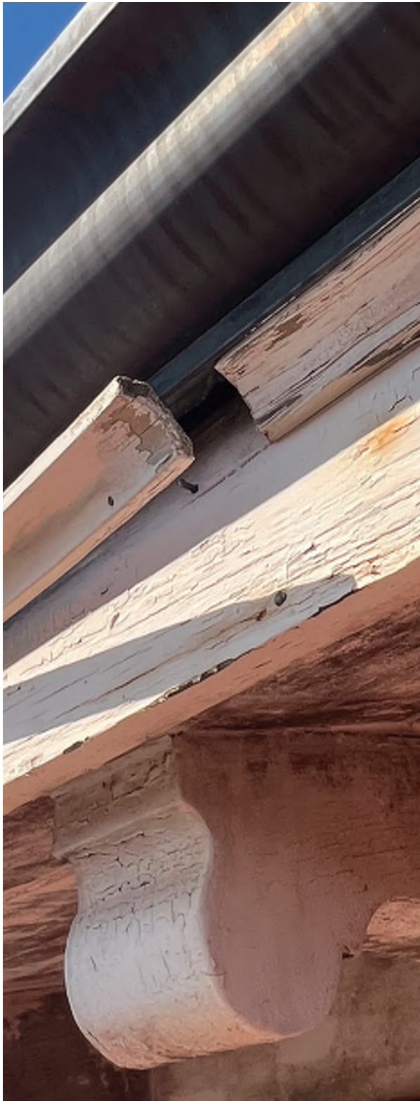
Image C-39: Thin and inexpensive bedmoulds for the gutters have not stood the test of time since gutter installation.
