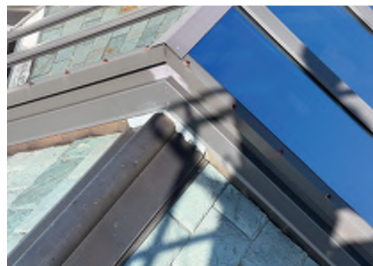
Image B-04: Heavily soldered joint where ridge cap meets the skylight and visibly open frame joint.
