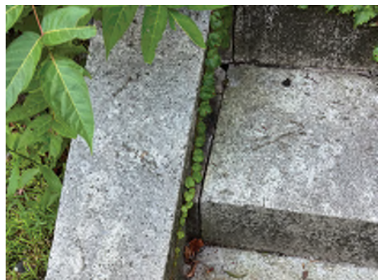
Image A-61: Wide cracking joint between the cheek wall and the granite steps. Vegetation is growing through the cracks.
