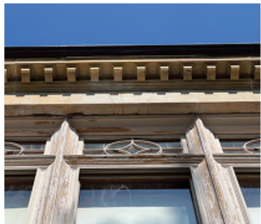
Image B-31: View of upper transom windows showing deteriorated caulking and brickmoulds.
