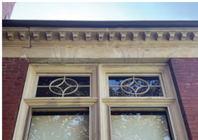
Image B-22: Deteriorated and cracked mortar joints at sandstone cornice caused by ineffective copper gutters and downspouts.
