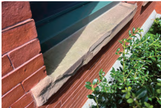
Image A-50: Cracking and spalling caused by the pressure of the load traveling down the edges of the masonry openings.
