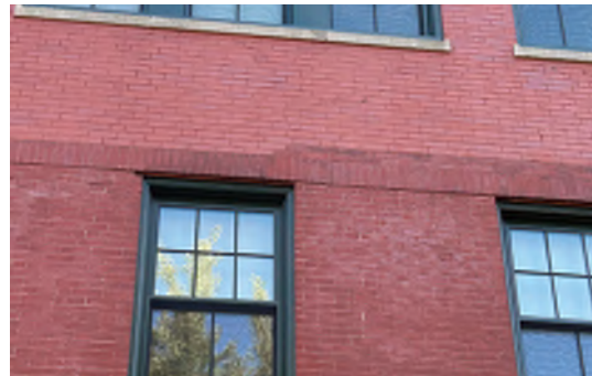
Image A-39: Area of bulging brick masonry at second floor window at north elevation due to rust jacking.
