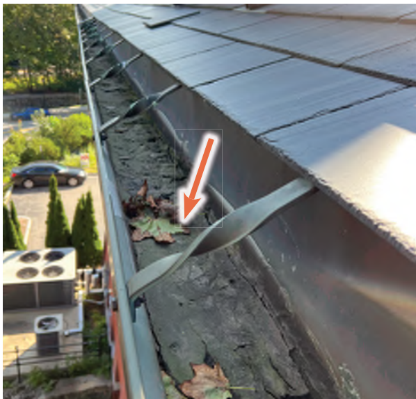
Image C-19: Compact gutter sediment and debris suggest improper pitch, allowing collection over time.
