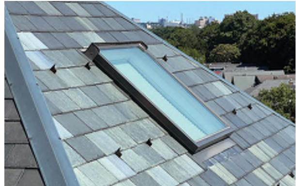
Image C-11: Modern skylight punctuate the slate roof in a few locations, with no reported leaking..
