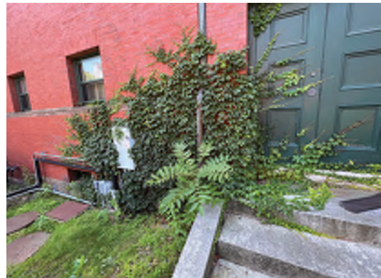
Image A-60: Vine overgrowth at brick masonry and granite stairs along the north elevation.
