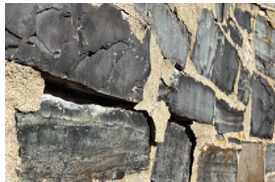
Image A-54: Bulging stone masonry at south retaining wall. Mortar is cracking and falling away from the stone.
