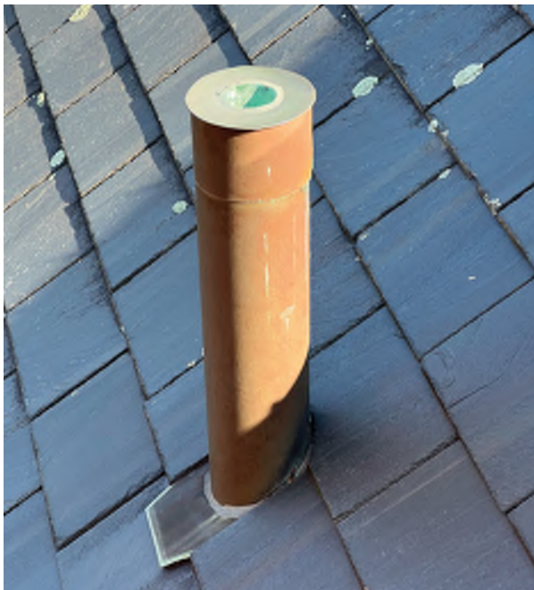
Image C-10: Copper vent pipes are in good shape, well-flashed, with solder joints intact.
