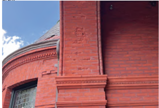
Image A-25: Isolated spalling at the west side of the intrados of the main entry arch.
