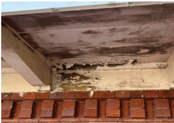
Image C-35: Flaking paint is prevalent at sites where water has entered the cornice and framing.
