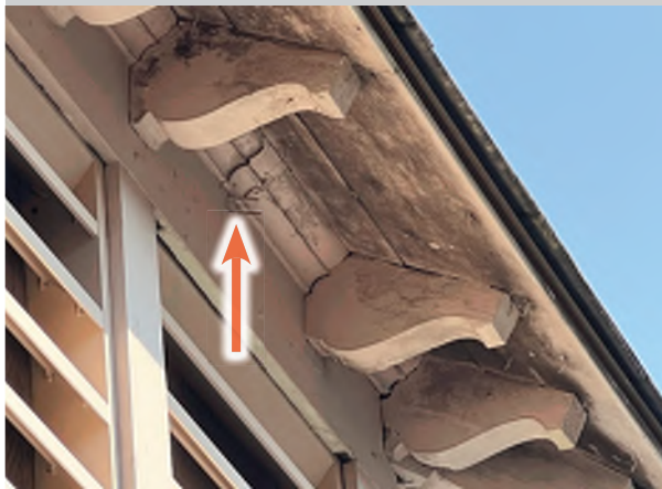
Image C-29: Missing brackets at the ventilator towers require replacement, and repainting overall.
