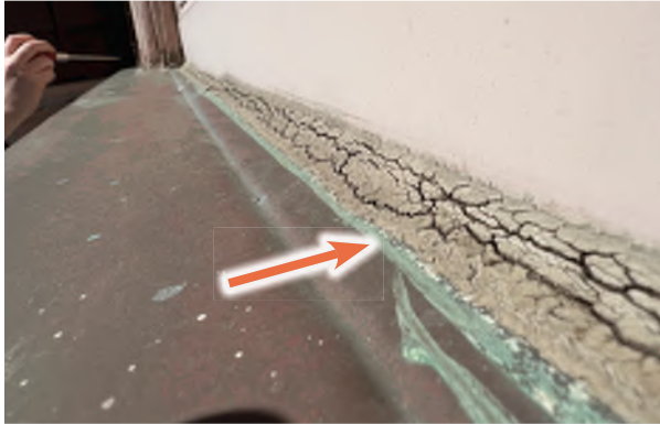
Image C-33: Cracked sealants between aluminum or vinyl windows and copper require replacement overall.
