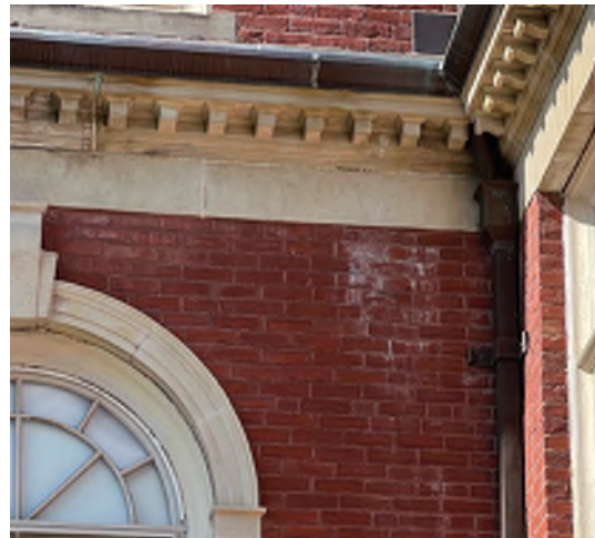
Image B-23: Staining and efflorescence at sandstone cornice and brick masonry caused by leaking gutter and downspout.
