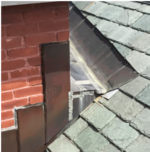
Image B-13: Vulnerable flashing transition at the southeast corner of elevator override. Broken seams, open joints, etc.
