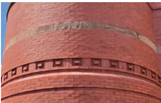
Image A-31: View of brownstone and brick banding at the turret. Note the erosion at the brownstone band.
