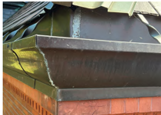
Image A-18: Typical k-style copper gutter at south west corner of the Town Hall. Note the open miter joint.
