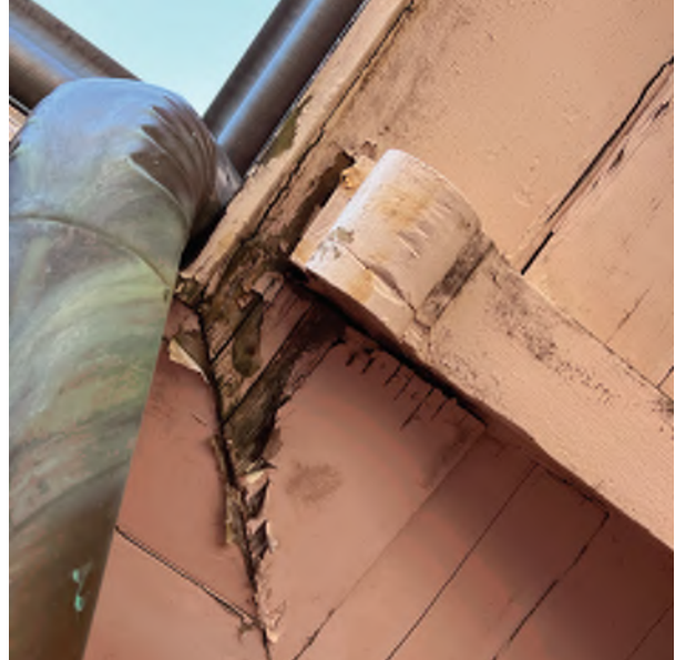
Image C-36: The worst of the cornice damage occurred at the inside corners of gutters where water is unimpeded.
