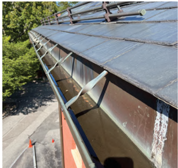
Image C-18: Ponding water in the gutters suggest improper drainage pitch.
