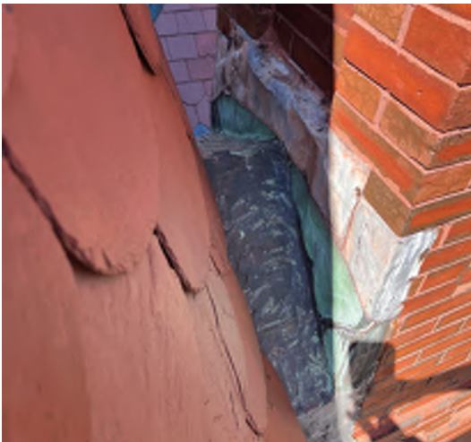
Image A-16: Deteriorated copper cricket and flashing between the turret and chimney. Heavily coated with mastic.
