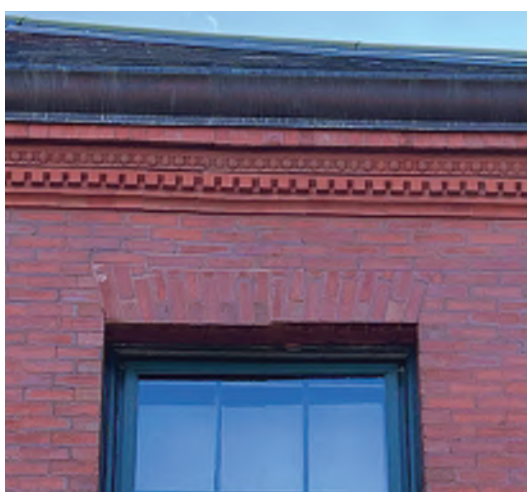
Image A-23: Slipping jack arch and step cracking at the second floor window at north elevation .
