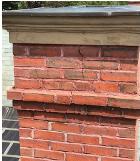
Image B-12: Significant structural cracking at the top of the south chimney. Note the deteriorated capstone.
