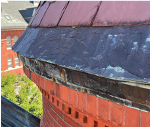
Image A-15: Heavy mastic wash over deteriorated copper skirt at the base of the turret roof.
