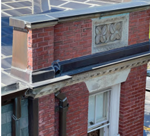
Image B-20: Through-parapet drainage detail suspected of compromising/damaging brick and sandstone masonry.
