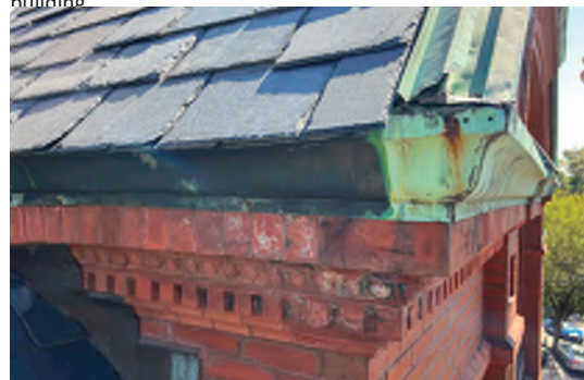
Image A-11: Damaged decorative brick cornice as a result of deteriorating copper and face nailing.
