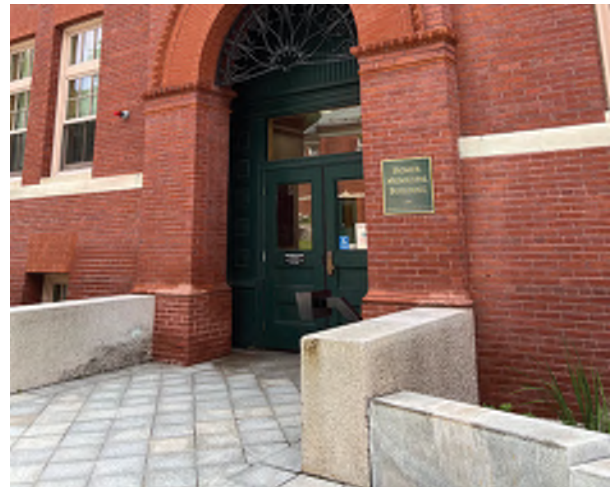
Image C-58: Similar rotating granite cheek walls have damaged the west entry brickwork as well..
