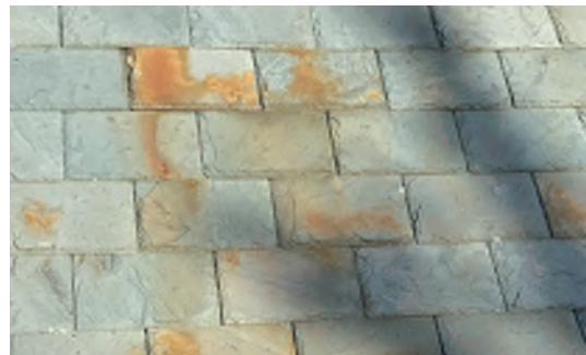
Image B-03: Oxidized slates at original slate roof on School Administration Building.
