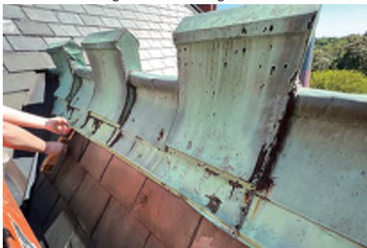
Image A-07: Ferrous nails were driven through the crestring to attach it to the roof. Mastic used to seal broken seams.
