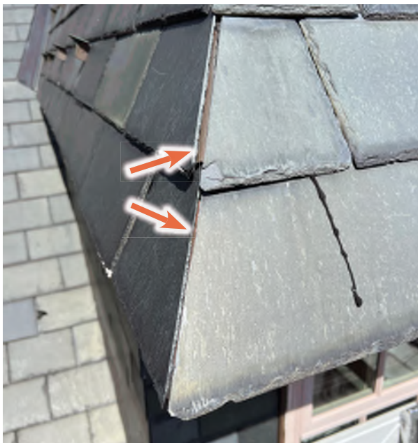
Image C-08: Interwoven flashing between the slate courses on the dutch gable dormer is a quality detail and water-resistant.
