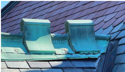
Image A-06: Original crenelated copper crestring is in poor condition due to age and weathering.
