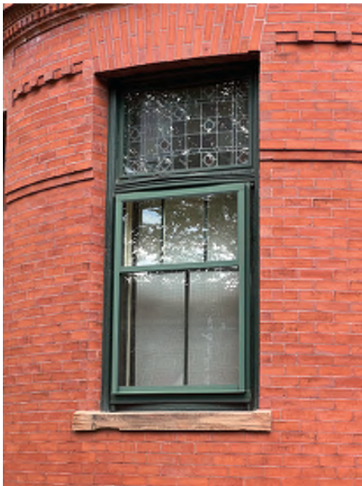
Image A-44: View of original wood window at south projecting window bay with stained glass transom.
