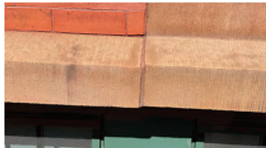
Image A-40: Movement at the modified brownstone lintel at the south elevation due to rust jacking
