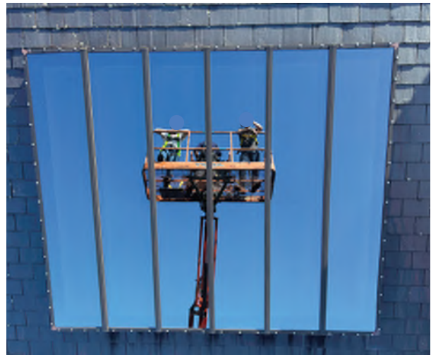
Image C-12: A large, generous modern skylight adorns the north roof slope, with no visible damage or compromised flashing.
