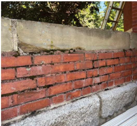
Image B-27: Severely deteriorated south site wall caused by water infiltration through sky-facing joints.
