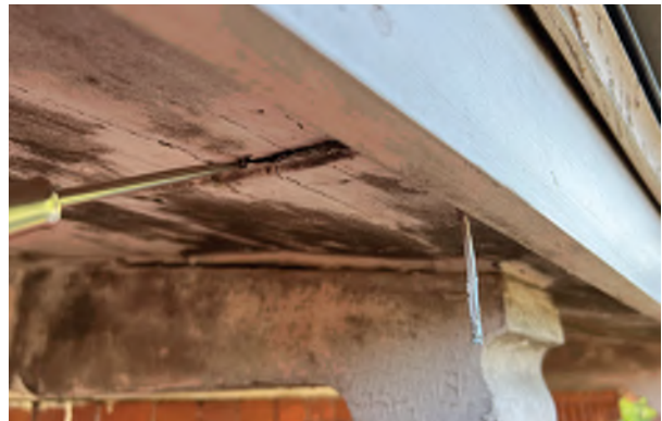
Image C-37: Soft end grain at soffit boards are pierced easily by an awl, suggesting they have been damp for some time.
