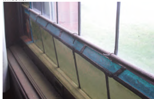
Image A-48: Buckling and deteriorated lead joints at large stained glass windows at the west elevation.
