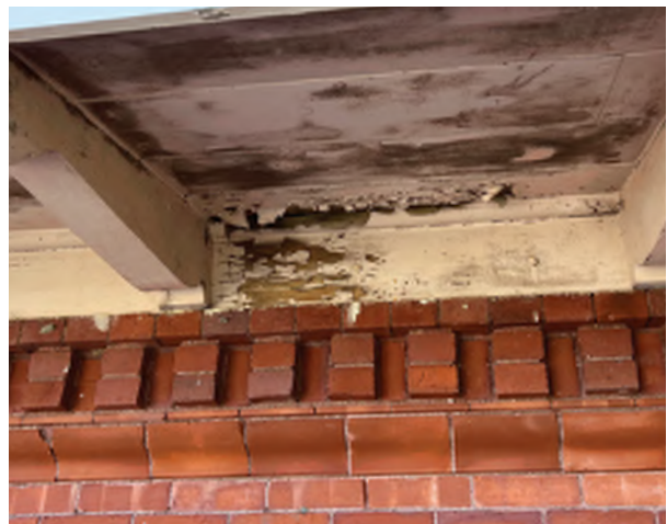
Image C-50: Brickwork at the eaves share in the suffering experienced by their wood cornices above, where water enters.
