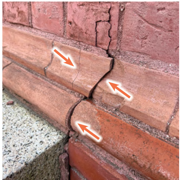
Image C-57: Upward thrust of the rotating granite cheek walls have cracked the brickwork at the intersection, consistently.
