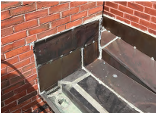
Image B-15: Poorly detailed copper counterflashing detail at chimney. No visible clips and new sealant joints required.
