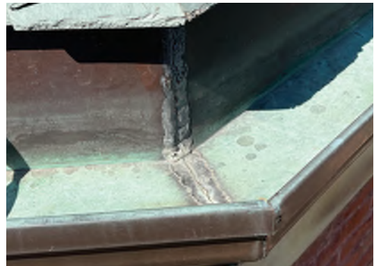
Image B-17: Broken solder seam at mitered corner of copper gutter.
