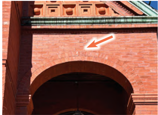
Image A-24: Slipping round arch and step cracking at the south portico. Note the broken keystone at the center of the arch.
