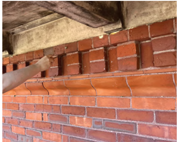
Image C-49: Some brickwork at the eaves are intact, still with their red-tinted mortar.
