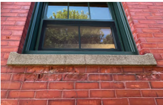
Image A-38: Spalling at brick masonry below the cracked first floor cast stone window sills at the north elevation.
