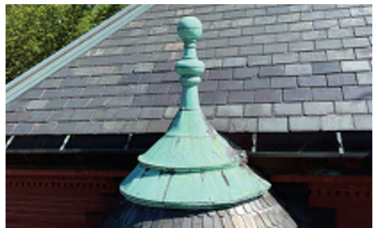
Image A-12: View of severely deteriorated original copper finial at south projecting bay window.
