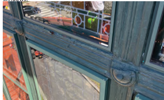
Image A-47: View of the deteriorated wood trim and bullseye rosettes at the south gable end's stained glass windows.
