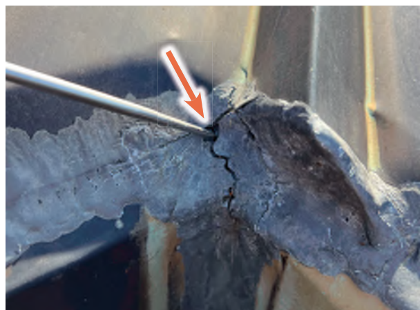
Image C-25: Large cracks at the intersection of copper valleys and gutters allow considerable water to enter and rot the woodwork.
