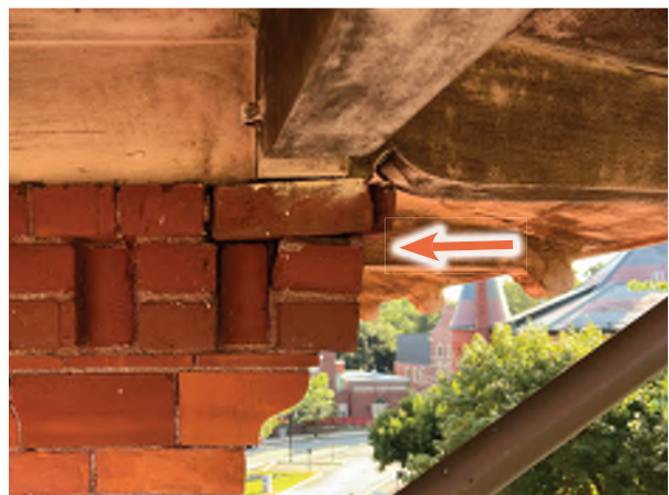
Image C-51: Loose bricks, notably at outside corners, require re-setting.
