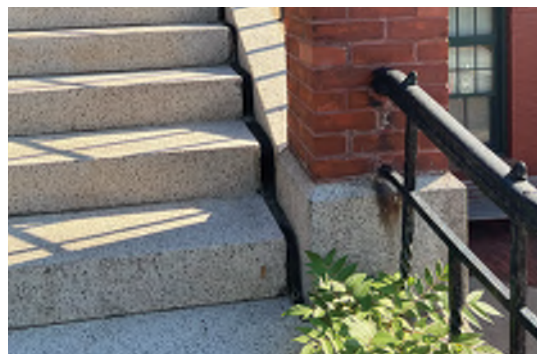
Image A-55: Wide cracking joint between the cheek wall and the granite steps at south portico infilled with sealant.
