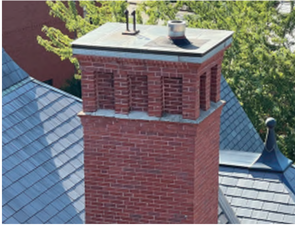
Image C-43: The building's solid brick chimney is plumb and intact, and appears to be well-capped.
