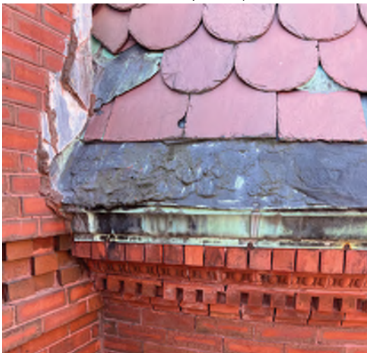
Image A-17: Severely deteriorated copper skirt, cornice, and flashing turret roof and chimney.
