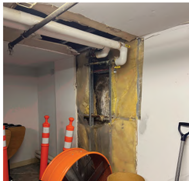
Image C-60: Internal leaks below the west entry suggest that water both ponds and enters the foundation..
