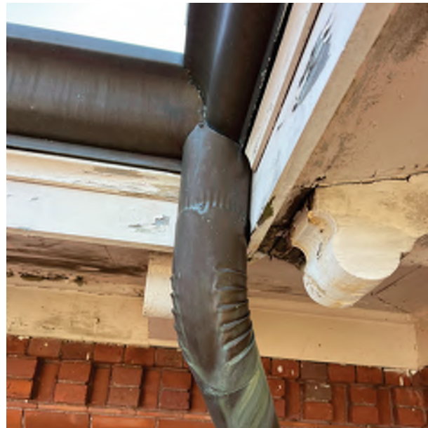
Image C-26: Copper downspout elbows are intact and appear to perform as they should.
