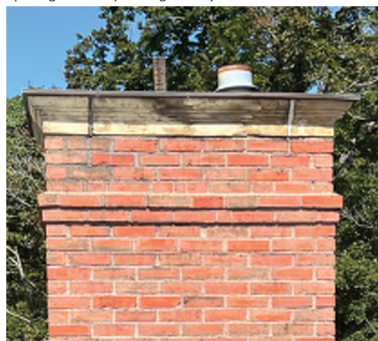
Image B-25: Deteriorated capstone at chimney.
