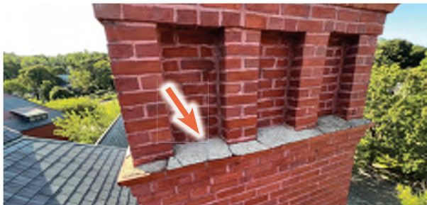
Image C-44: A deteriorating mortar wash at the chimney should be replaced to ward off standing water.
