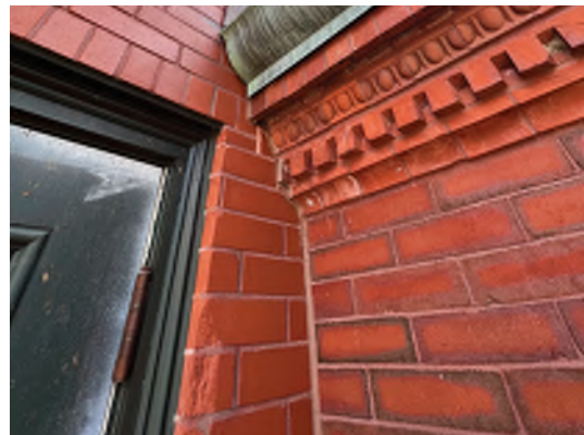
Image A-42: Spalling and deterioration of the masonry opening around the door to the fire escape.
