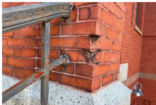
Image A-57: brick deterioration caused by twisting metal handrails as a result of the failing retaining wall.
