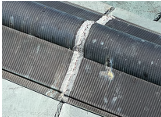
Image B-05: Broken solder seam at ridge cap. Copper appears to be in otherwise good condition.
