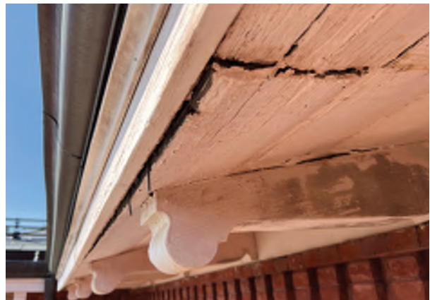
Image C-38: The worst of the woodwork is easily visible from below, requiring replacement.
