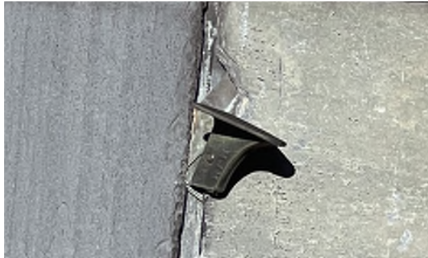
Image C-14: Bent retro-fit snowguard pads are prevalent and generally ineffective at snow-retention.
