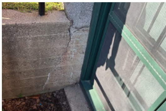
Image A-59: Crack at the concrete window well wall at the foundation on the south elevation.
