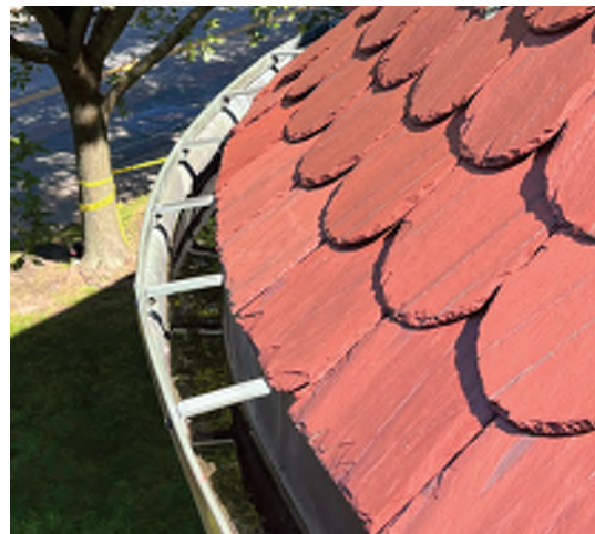
Image A-19: Water and debris collecting in the gutters away from the downspouts, suggesting an issue with the pitch.
