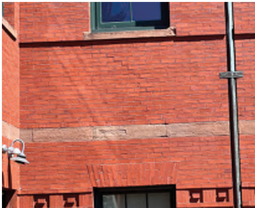
Image A-21: Slipping jack arch and step cracking at ground floor windows at south elevation
