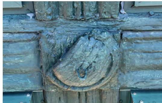
Image A-46: View of the deteriorated wood trim and bullseye rosettes at the south gable end's stained glass windows.
