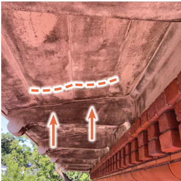
Image C-34: Cupping soffit boards suggest they have been damp in years past, possibly due to low-quality woods used in replacement..
