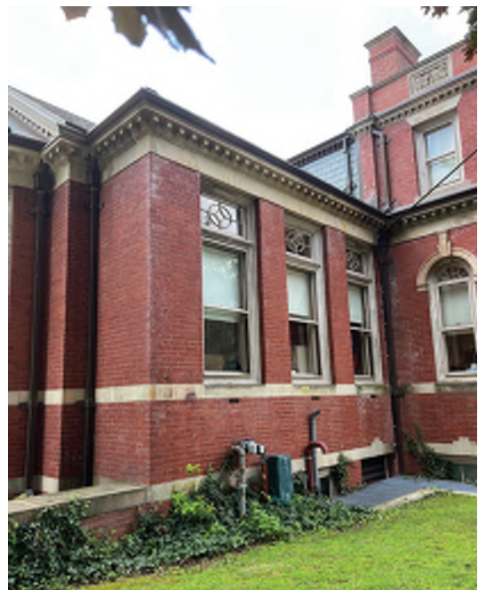
Image B-18: View of northwest corner of the building showing deterioration to sandstone cornice and brick masonry.
