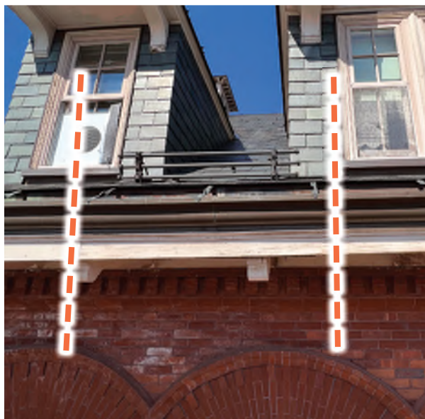
Image C-16: Wood and masonry deterioration appear to related directly to snowguard fences in areas between dormers.
