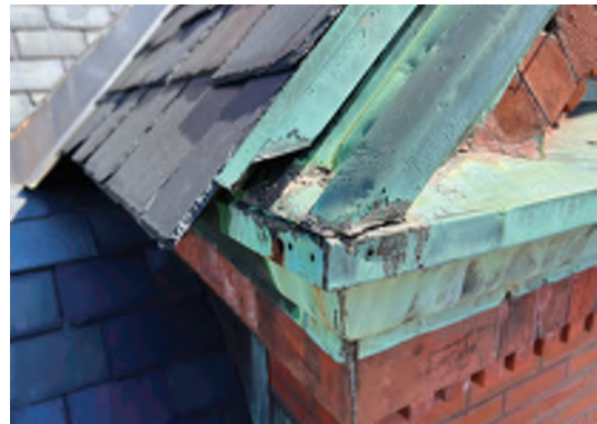
Image A-10: View of deteriorated decorative copper moldings at the south gable end. Condition is typical across building.
