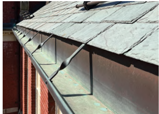
Image B-16: Approx 20 year old copper downspouts in good condition. No corrosion, pinholes, or metal deterioration.
