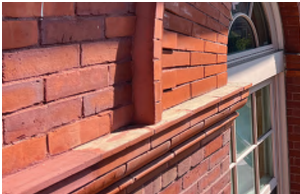
Image C-54: Elsewhere on the same projecting stringcourse, a missing mortar wash should be reestablished.
