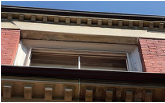
Image B-26: Bulging lintel at top floor or east projecting bay.
