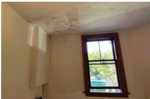
Image B-08: Interior damage at southwest stairwell caused by chronic roof leaks.
