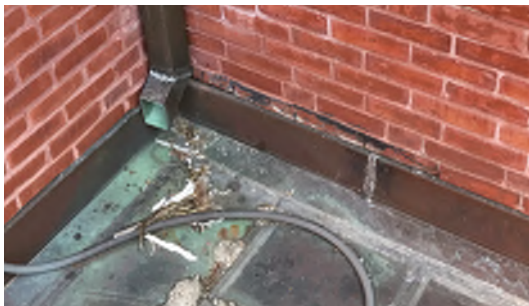
Image B-07: Open mortar joint at reglet of east portico counter flashing. Requires new urethane sealant joint.
