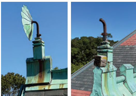
Image A-09: View of the original copper floral finial at the west gable end (Left) and the missing finial (Right)
