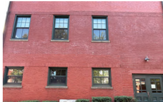
Image A-41: Efflorescence appears to be more prominent at second phase of addition.
