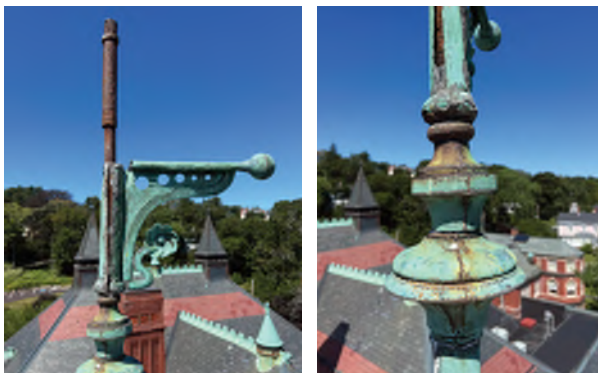
Image A-14: Significantly deteriorated original copper weathervane at the top of the turret. Much of the weathervane is missing.
