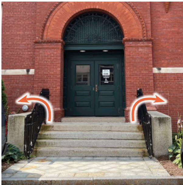
Image C-55: Rotating granite cheek walls at the north entry have slowly wreaked havoc on their adjacent bricks at the building.
