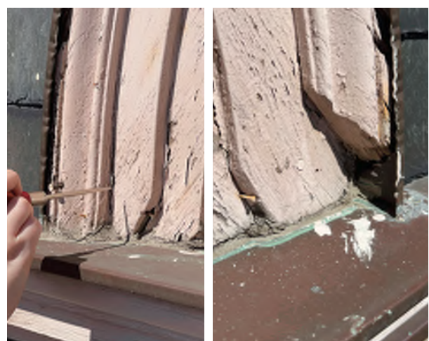
Image C-32: The arched dormer window casings would do well to receive epoxy consolidation for prolonged life.
