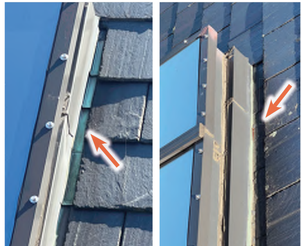
Image C-13: The large modern skylight appears to sit on an older copper curb, intact and without reports of leaking.
