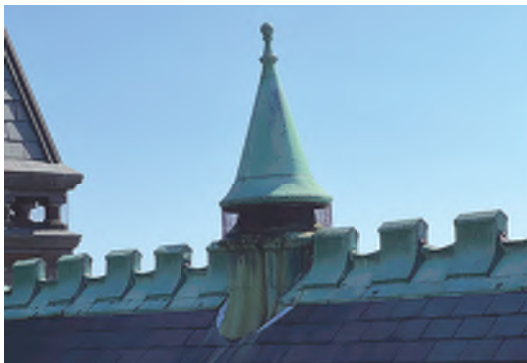
Image A-08: View of copper ventilation cupola integrated with the crenelated crestring at the north-south ridge.
