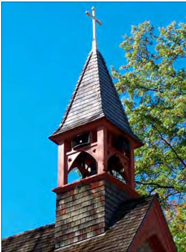
Figure 2. Example of shingle siding after many years of service.
