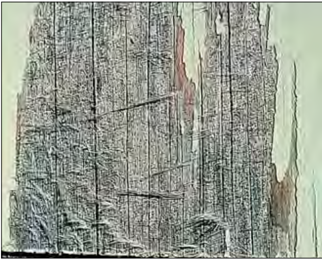
Figure 17. Severely weathered wood surface.
