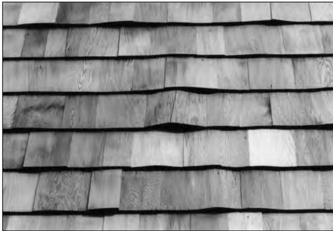
Figure 7. Buckling of shingles installed with insufficient gap.
