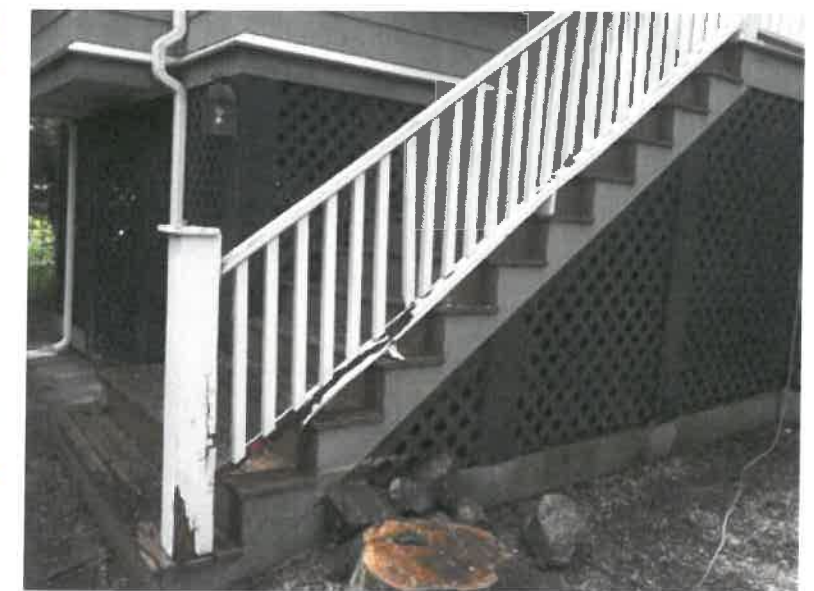
EXISTING STAIR ALSO ROTTED AND UNSAFE
