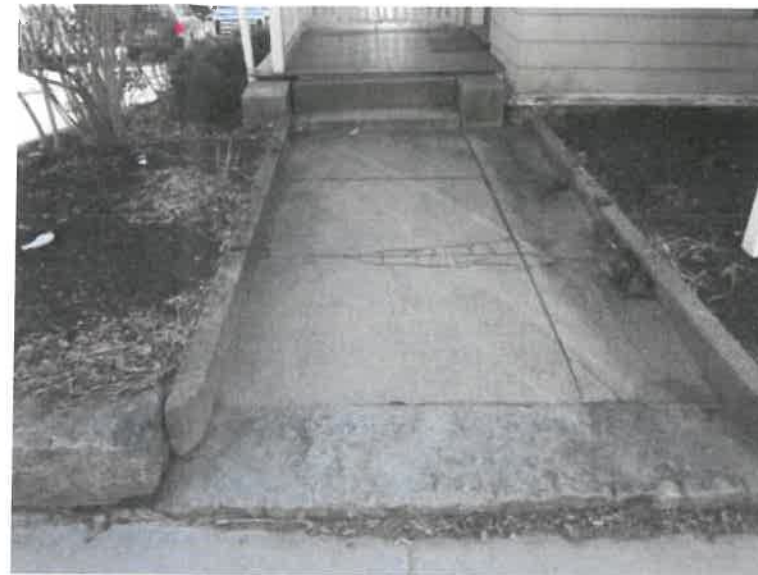
ENTRANCE WAY IS COMPROMISED OF CRACKED AND LOPSIDED CONCRETE AND IS OFF CENTER WHEN LEADING TO WEAKENED WOODEN ENTRANCE PORCH.
