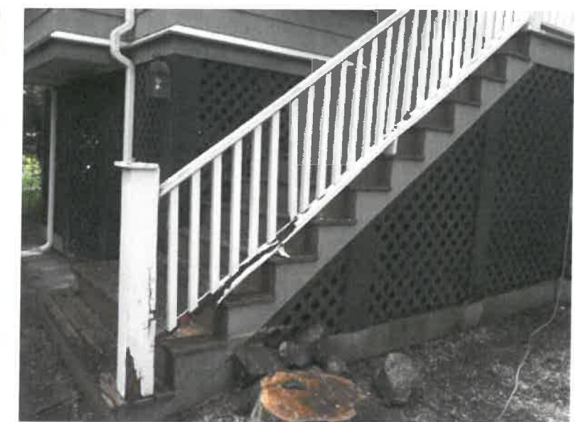
EXISTING STAIR ALSO ROTTED AND UNSAFE
