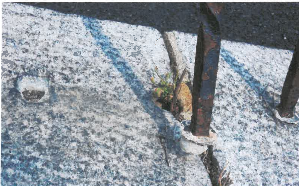
2. Close up view of railing pickets. Picket to the left is missing, center picket is bent and loose. Note lead around very shallow embedment of pickets.
