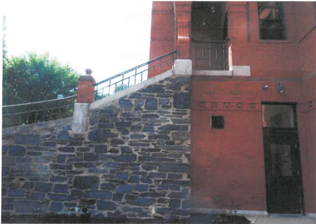
3. View of North end of the stone retaining wall showing connection with the buildings brick walls.
