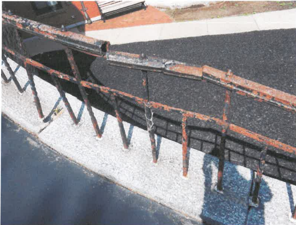
1. Close up view of railing showing broken top rail and ineffective attempts to weld.
