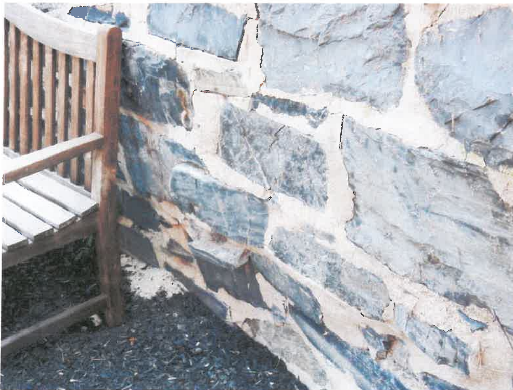
4. Close up view showing cracked mortar joints and displaced stone work.
