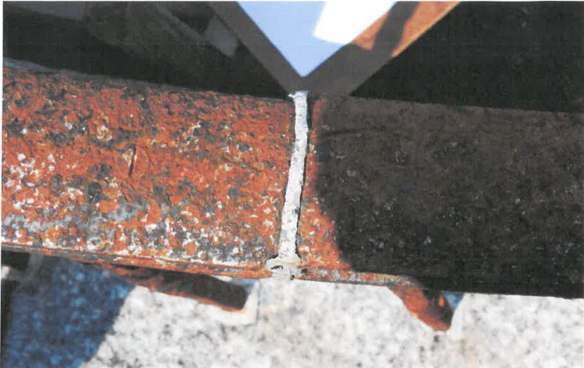
5. Close up view showing an original lead joint between sections of cast iron.
