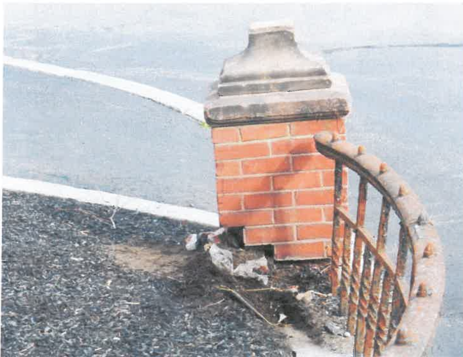
6. View of lower brick pier which has been knocked off of its foundation and is missing its spherical finial.
