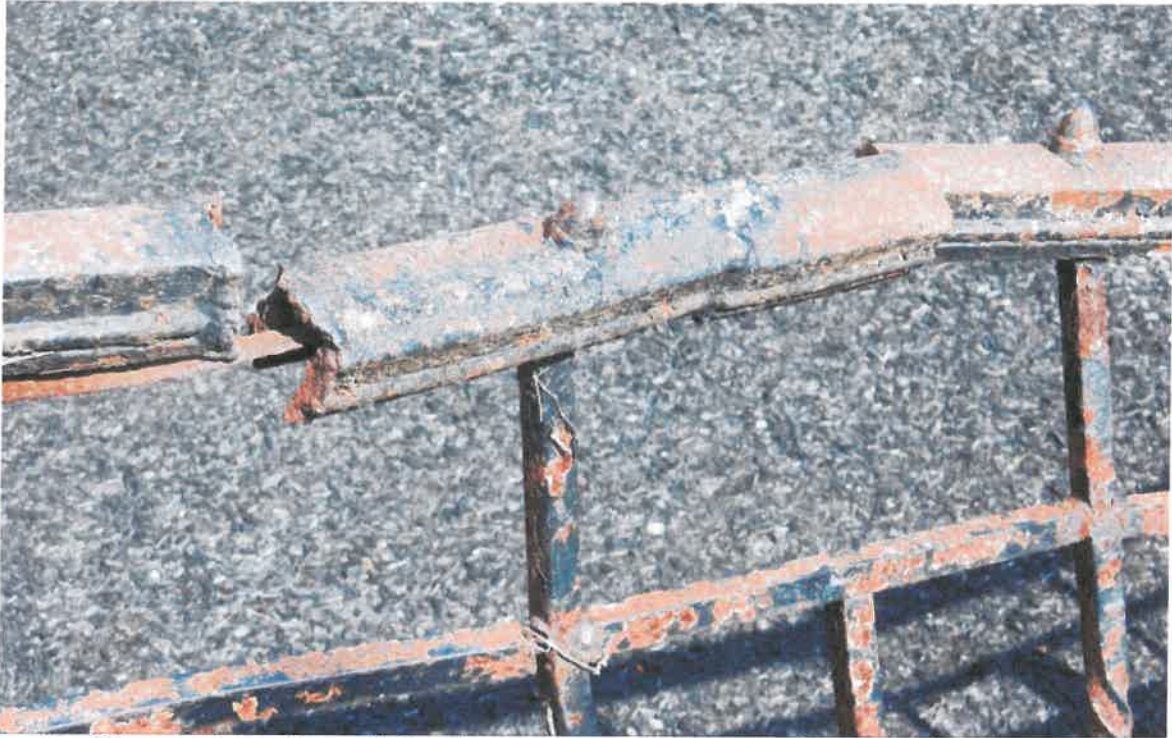
3. Close up view of top rail showing broken welds and severely rusted sub-rail.
