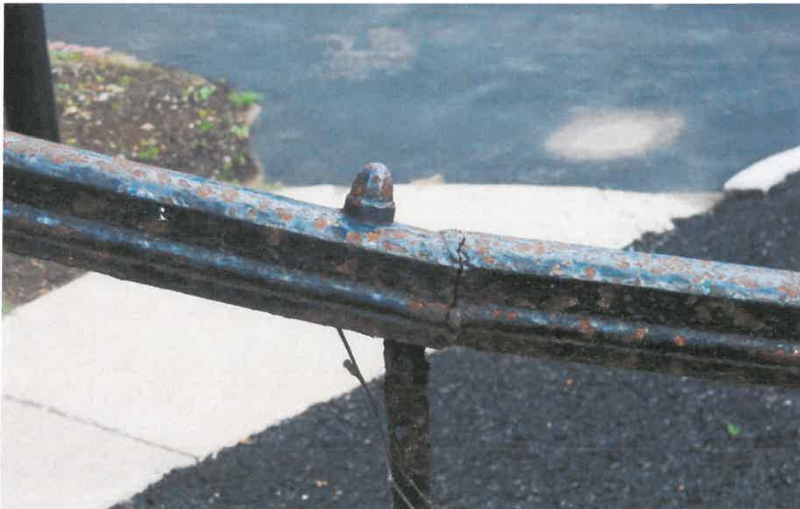
6. Close up view showing decorative (non-functional) bolts and broken weld.
