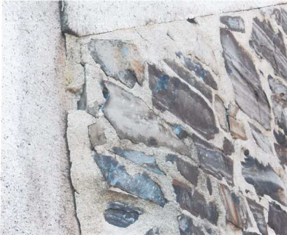
5. Close up view showing differential movement between granite pier and shale as well as between granite pier and granite coping stone.
