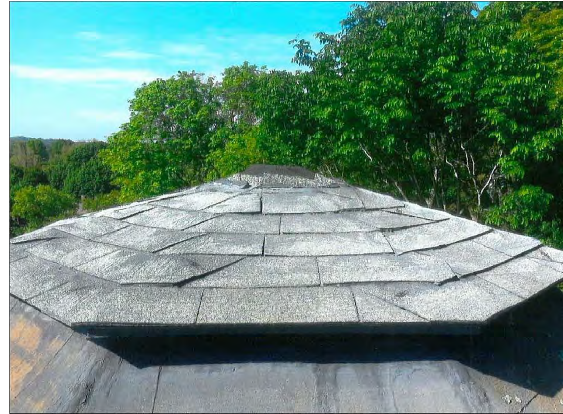
EXISTING CUPOLA WITH PATCHED FINIAL BASE AND DETERIORATED ROOF MEMBRANE
