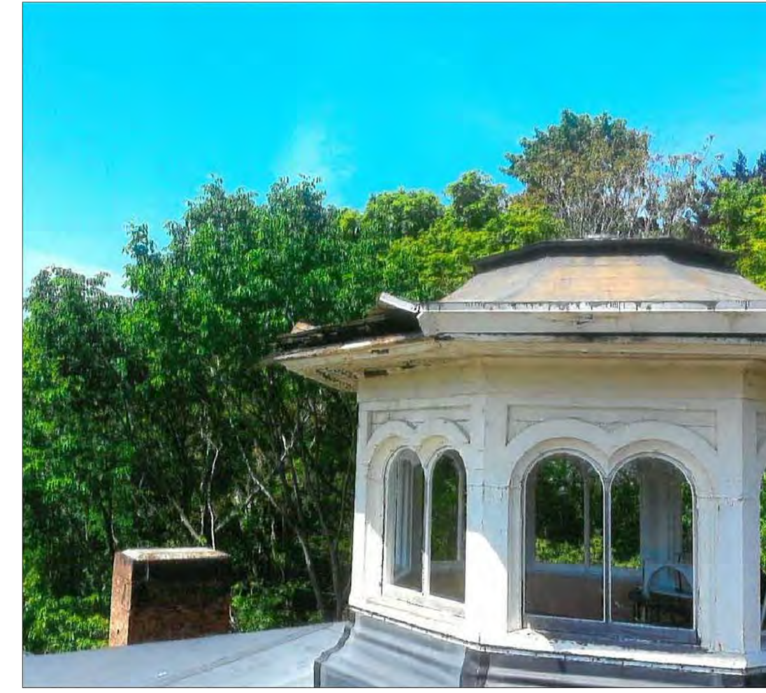
EXISTING CUPOLA WITH MISSING CORNICE AND FINIAL, SHOWING RUBBER ROOF COVERING BASE
