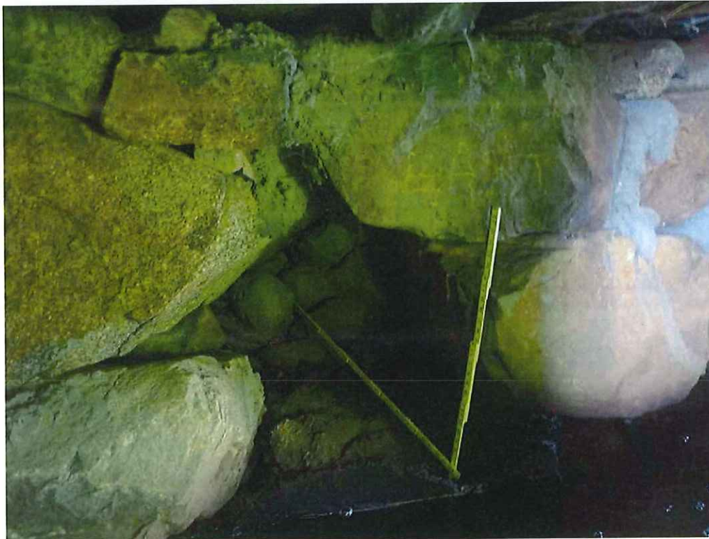
Photo 24: East Abutment below Slab 5 at the waterline: 2'-6" L x 2'-3" H x 3'-2" D void.
