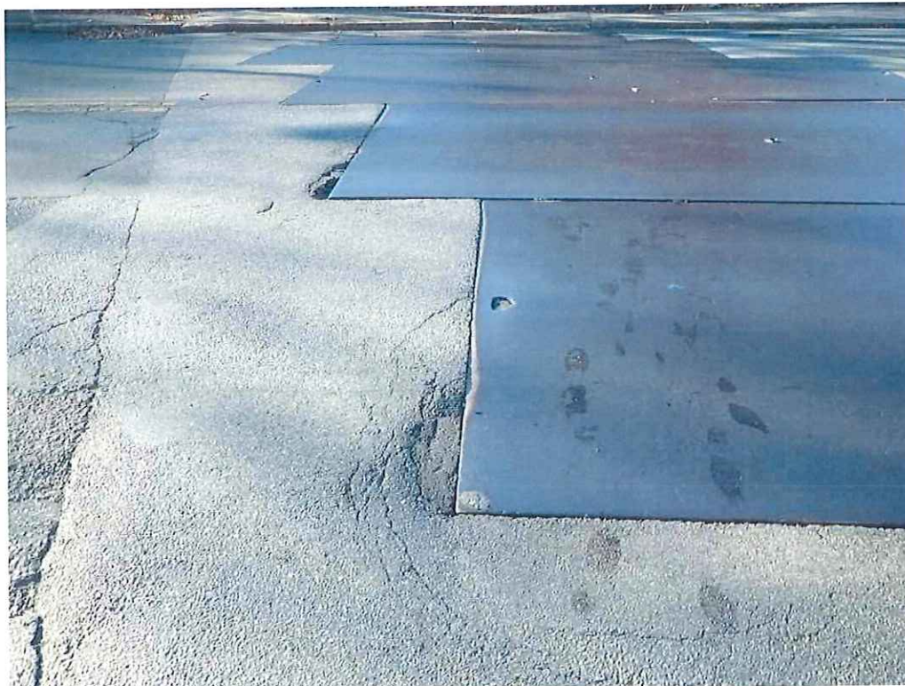
Photo 14: Steel Plate 4 and 5 at the northeast corner have 2'-4" W x 7" L x 2" D spall and 2'-0" W x 7" L patch with radial cracking, respectively.
