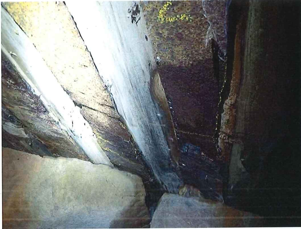
Photo 19: Steel Beams 2 and 3, bottom flange near East Abutment: Up to 100% section loss x 1" wide with 3/16" thickness remaining.
