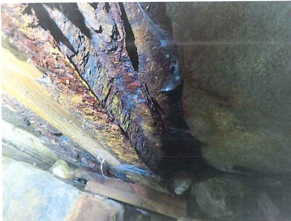
Photo 20: Steel Beam 8 bottom flange near Mid-span: 100% section loss x up to full width.
