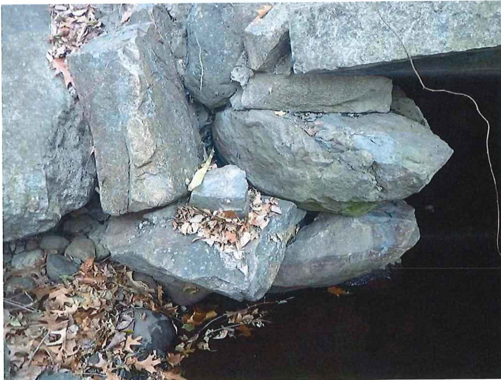
Photo 22: South face of West Abutment: 2'-0" L x 18" H x 14" D void with shifted stones
