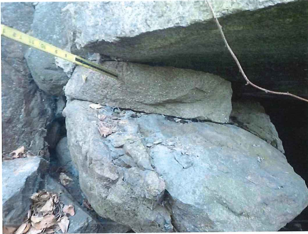
Photo 15: Slab 1 southwest corner at West Abutment: Slab is unsupported for 6".
