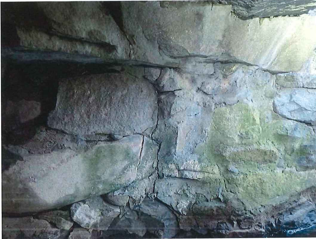
Photo 23: East Abutment below south edge of Slab 1: Multiple stones with vertical cracks up to 10" L x up to 1/4" W and an isolated 5" H x 1-1/2" W x 3" D spall.
