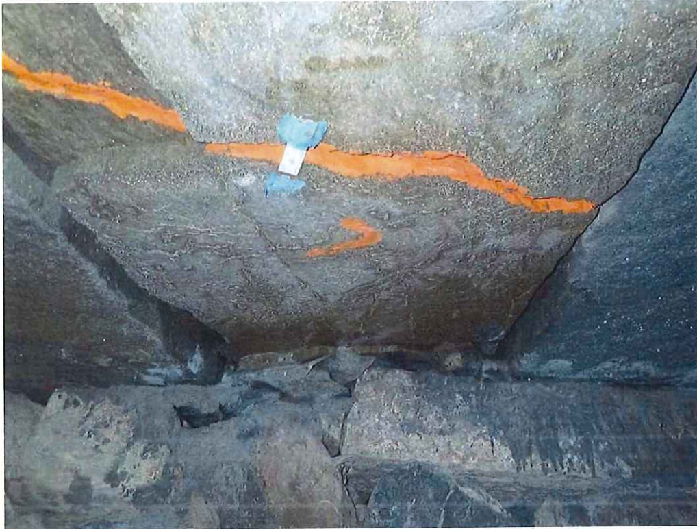
Photo 17: Slab 7 near Mid-span: Up to 2" W x FW x FD crack with a 20" L x 13" W x 2" D spall. Note: Crack gauge.
