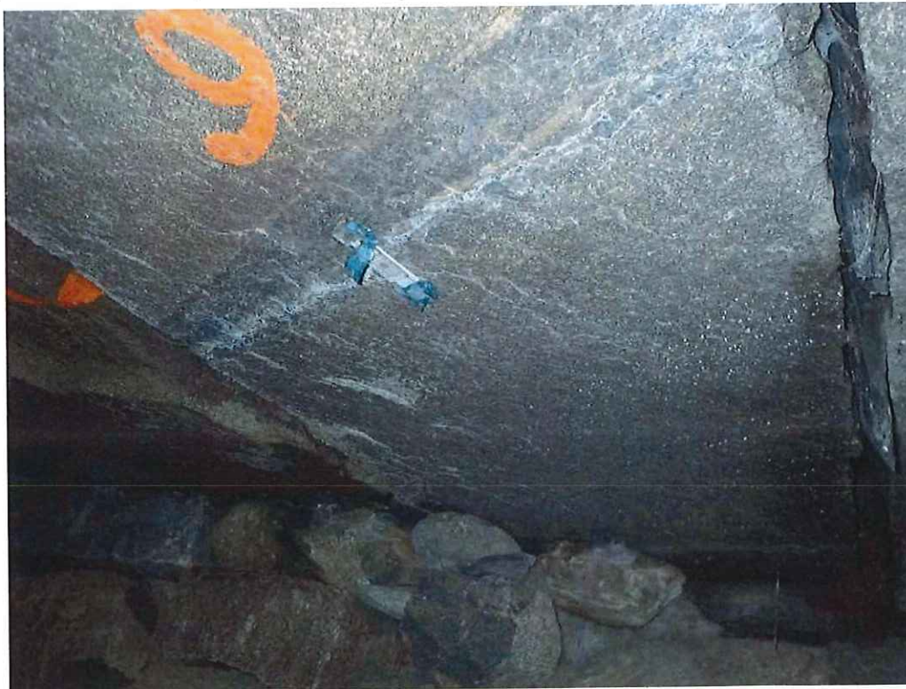
Photo 16: Slab 6 underside near Mid-span: Transverse hairline crack with efflorescence. Note: Crack Gauge.
