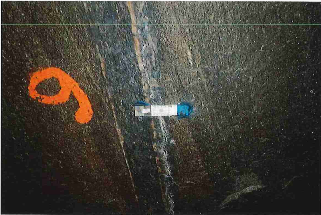
Photo 3: Granite Slab 6 - Split at mid-span.
