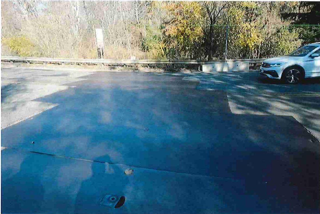
Photo 1: Typical condition of the steel plates. Note the height difference between P1 & P2 due to broken welds.
