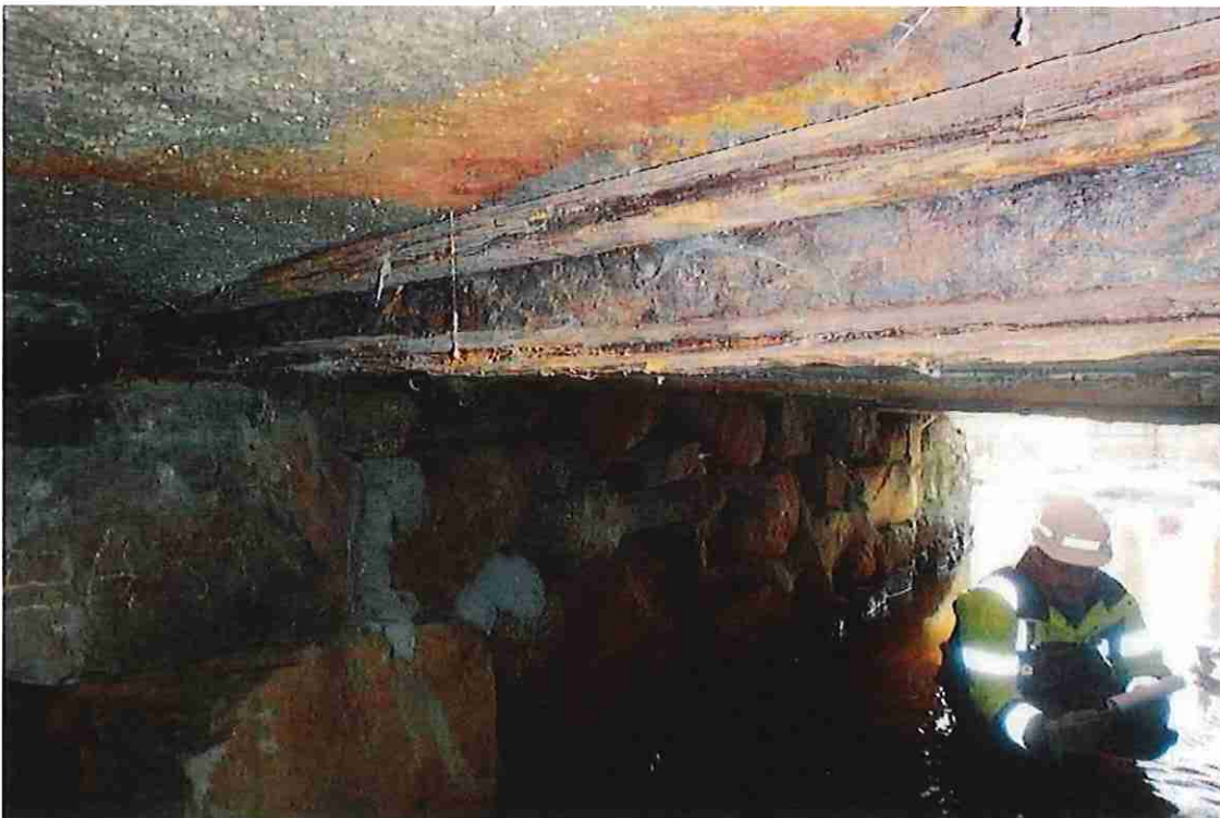
Photo 8: Typical heavy section loss and lamintination to the steel at the east end bottom flanges Northern side of Beam 8 shown.
