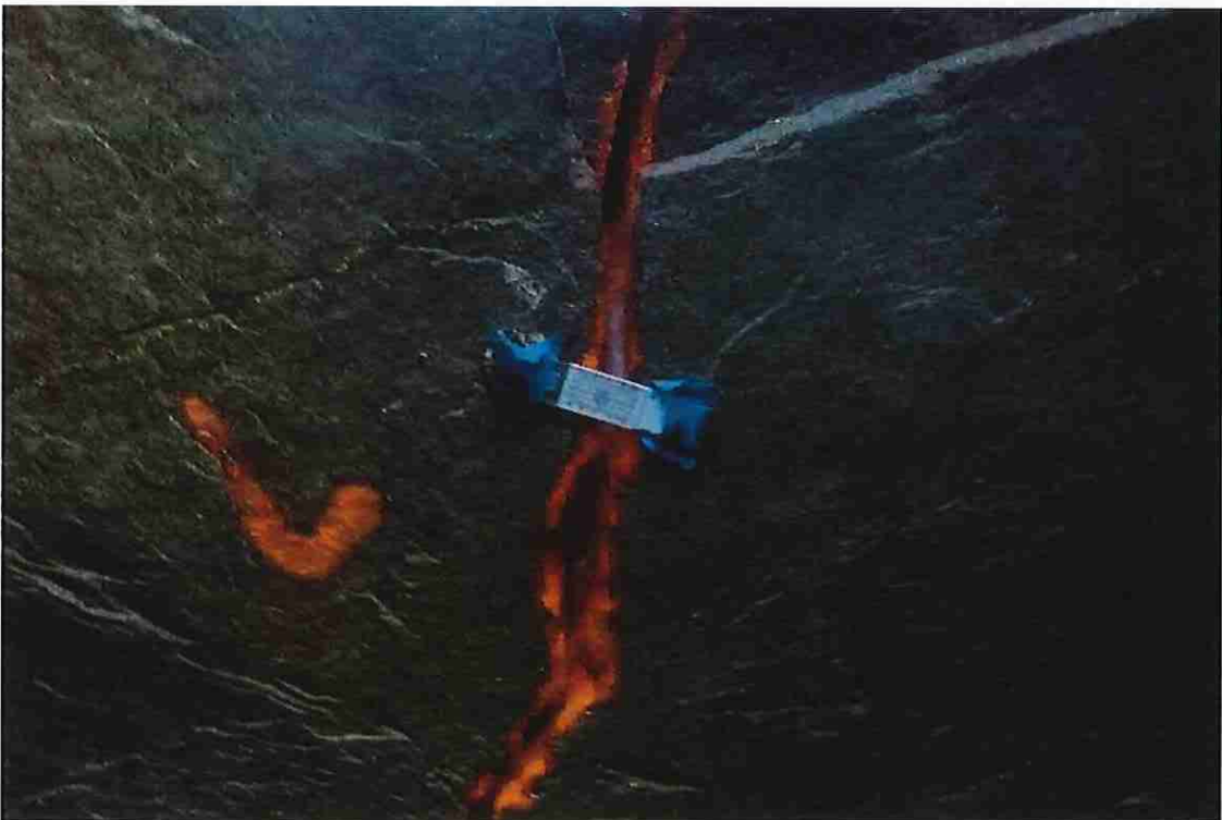
Photo 4: Granite Slab 7 - Split at mid-span.
