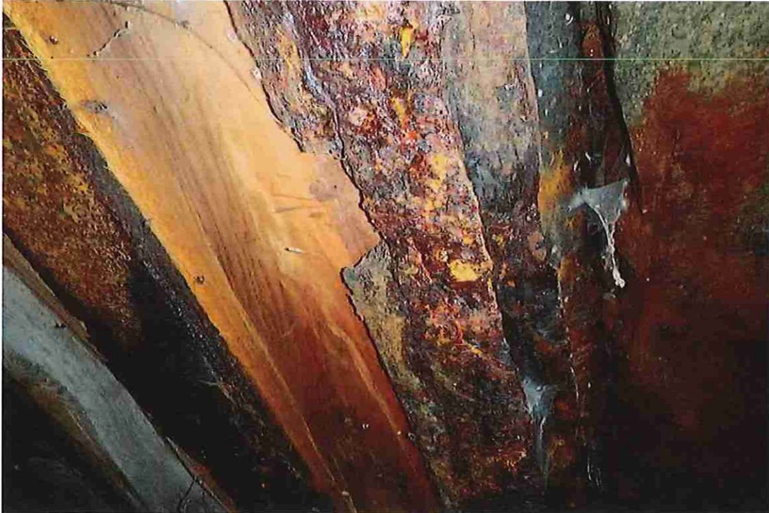
Photo 9: Heavy section loss up to 100% at the west end bottom flanges of Beams 7 (left) & Beam 8 (right).
