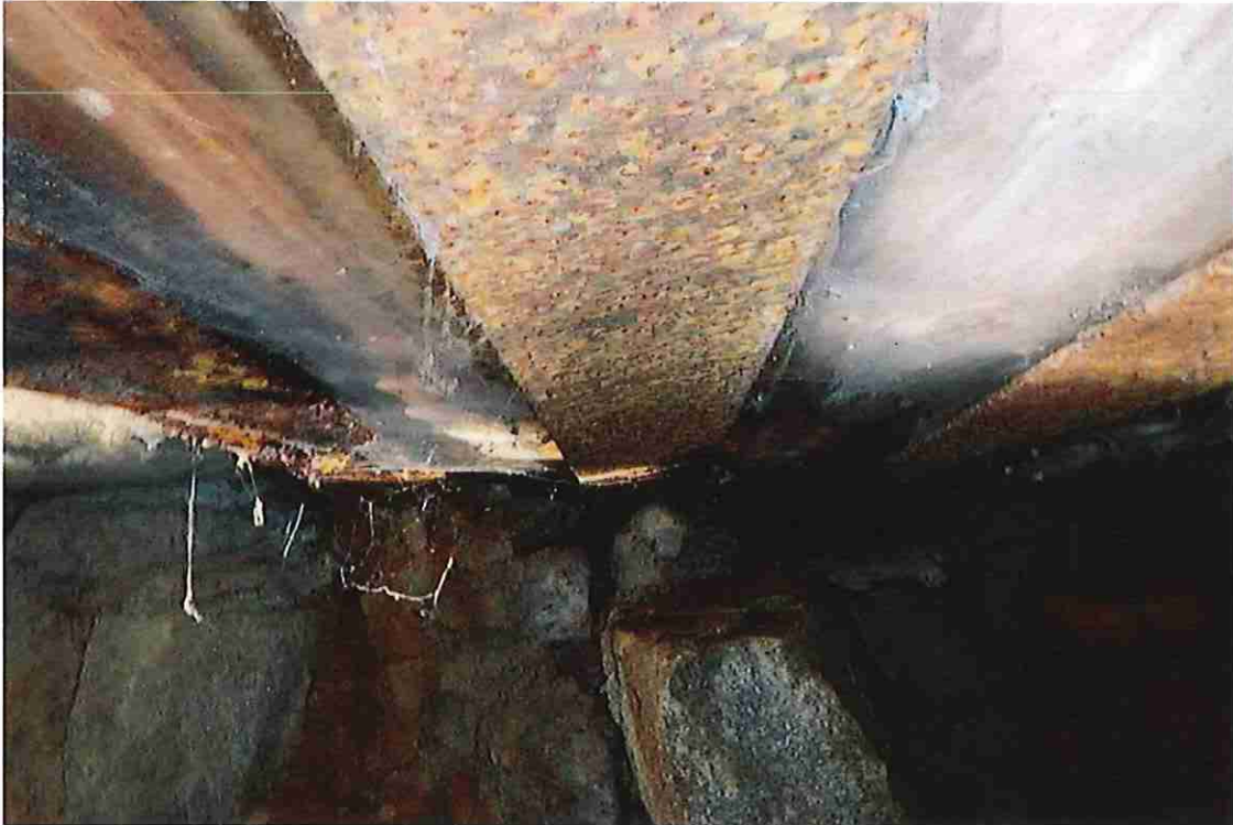
Photo 7: The beams typically exhibit minor rotation about the longitudinal axis, resulting in the bottom flanges no longer being level. Beams 1 - 3 shown. Note the timber shielding in between beams.
