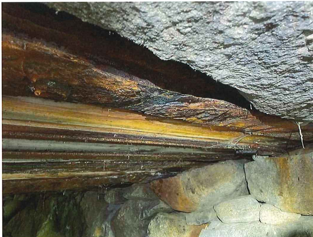
Photo 14: Steel Beam 1 bottom flange near Mid-span: 100% section loss x 1" wide at the south toe with 3/16" thickness remaining.
