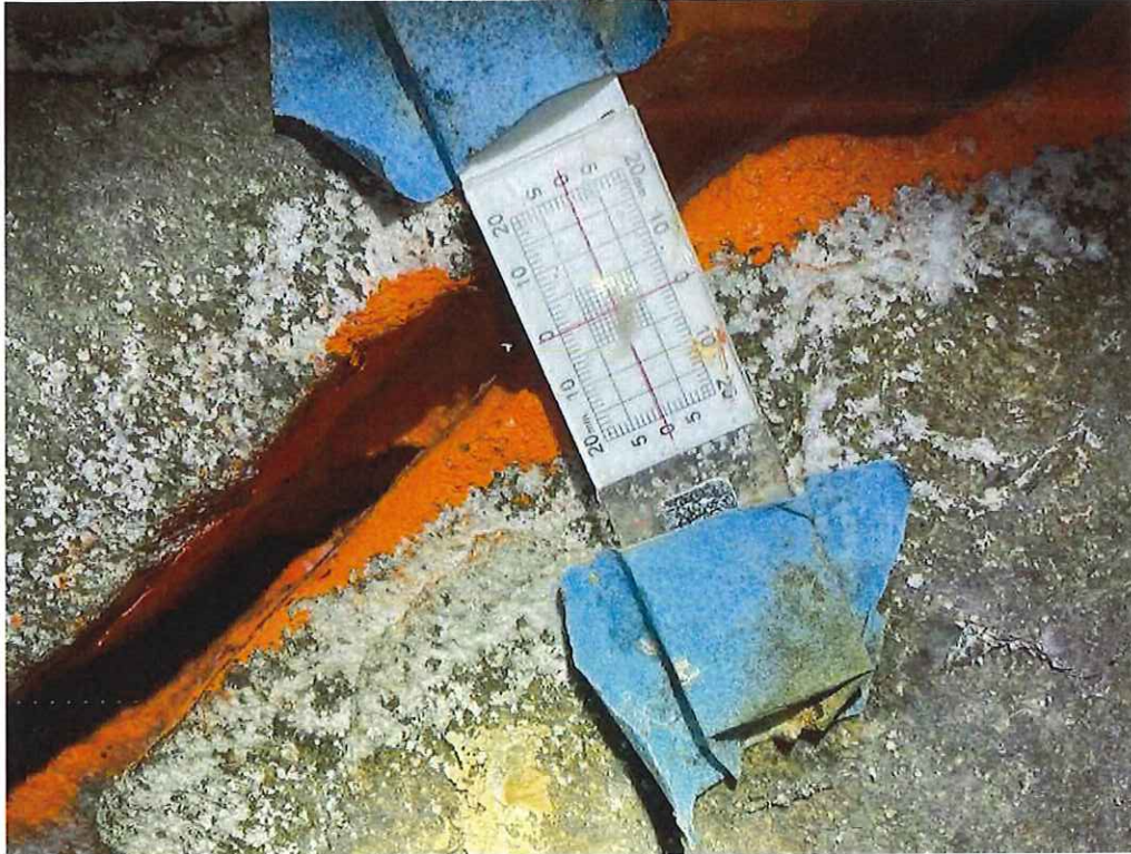
Photo 21: Slab 7 near Mid-span: Crack gauge shows minor movement ( < 1 mm in longitudinal direction only). No change since previous inspection.
