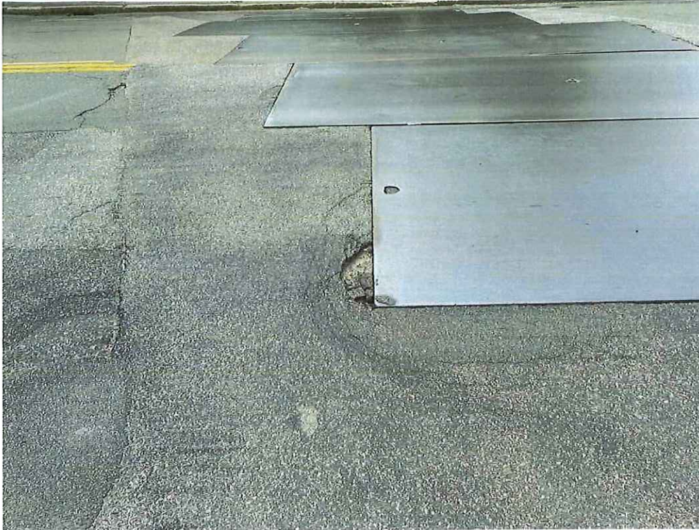
Photo 11: Steel Plate 5, northeast corner: 2'-0" wide x 7" long x up to 2" deep spall.
