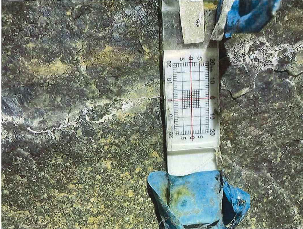
Photo 19: Slab 6 underside near Mid-span: Crack gauge shows minor movement ( < 1 mm in both directions). No change since previous inspection.
