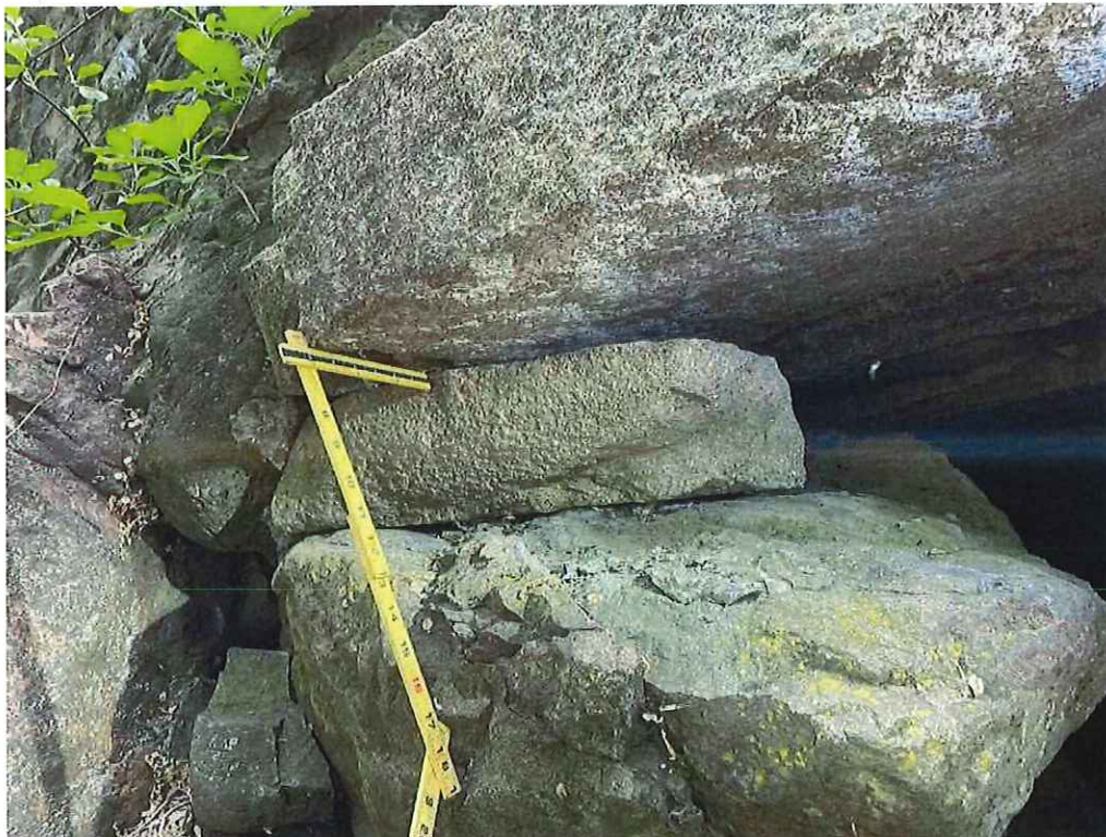
Photo 12: Slab 1 southwest corner at West Abutment: Slab is unsupported for 6".
