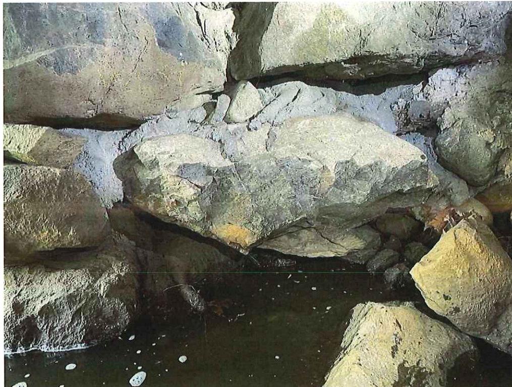
Photo 24: West Abutment below Slab 2: 3'-4" long x 20" high x 2'-0" deep void with shifted stones.
