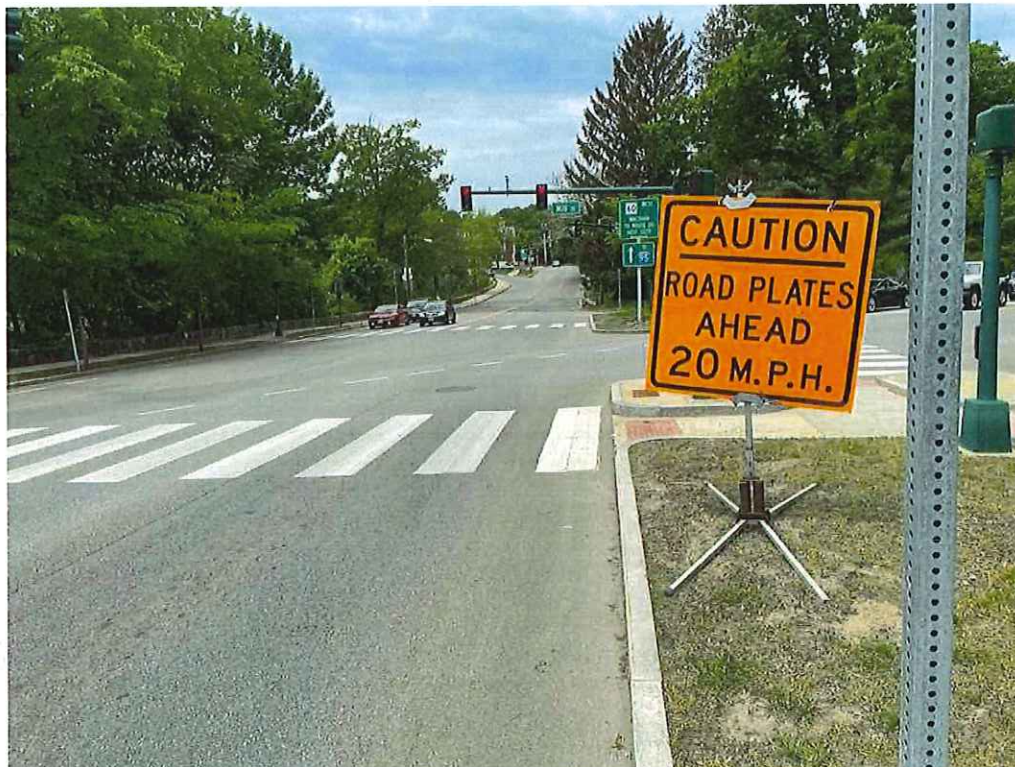
Photo 8: "Caution" sign in-place at the east approach
