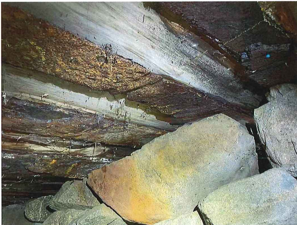
Photo 16: Steel Beam 3 bottom flange at West Abutment: 100% section loss x 1/2" wide at both toes with 1/8" thickness remaining.
