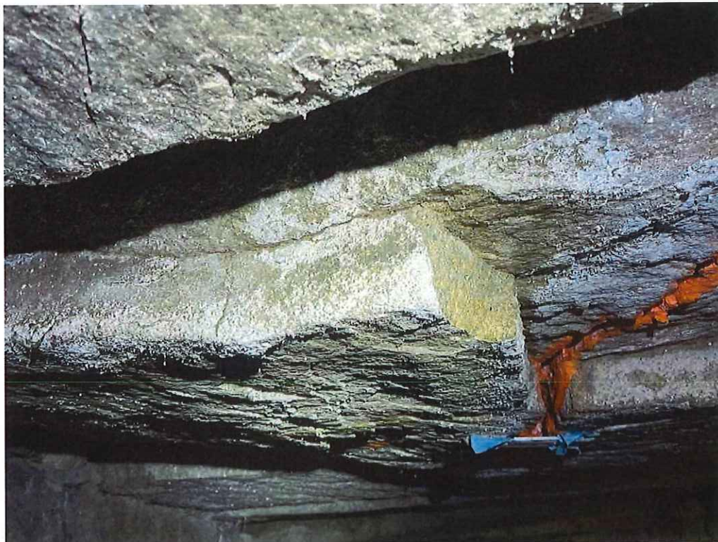
Photo 22: Slab 7 near Mid-span at the south edge: 20" long x 13" wide x 2" deep.
