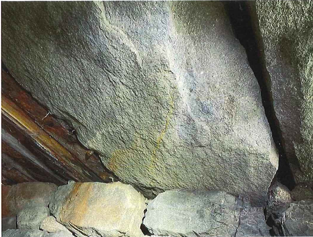
Photo 13: Slab 4 underside at East Abutment: diagonal hairline crack.
