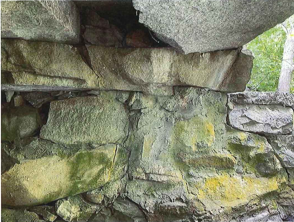
Photo 25: East Abutment below the south edge of Slab 1: Multiple stones with vertical cracks.
