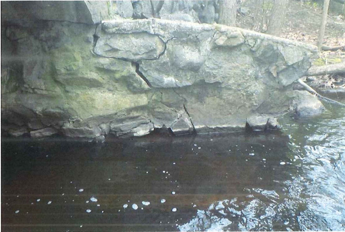
Photo 19: Southeast wingwall: Full height crack measuring up to 6" wide x up to 2' deep.
