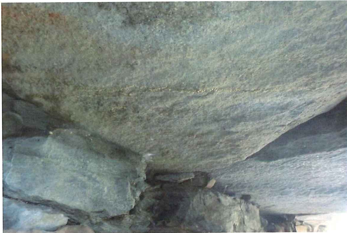
Photo 10: Granite slab 4: Diagonal hairline cracking at the east end.
