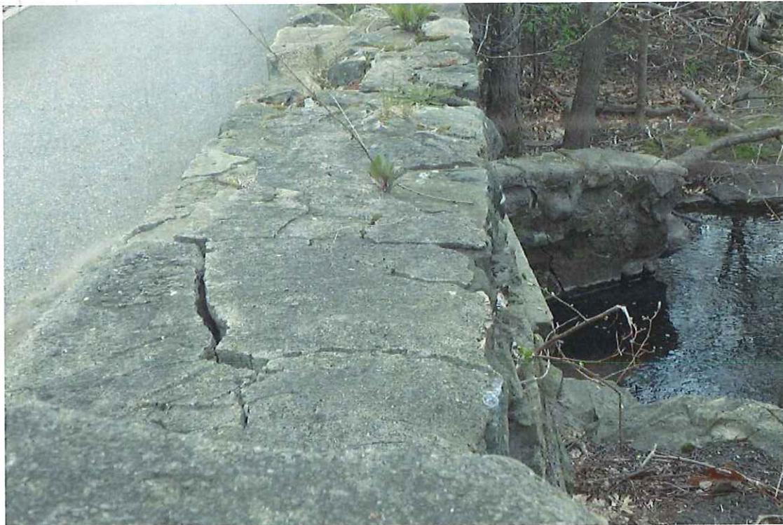
Photo 6: Bulging of western half of masonry wall along area of water intrusion.
