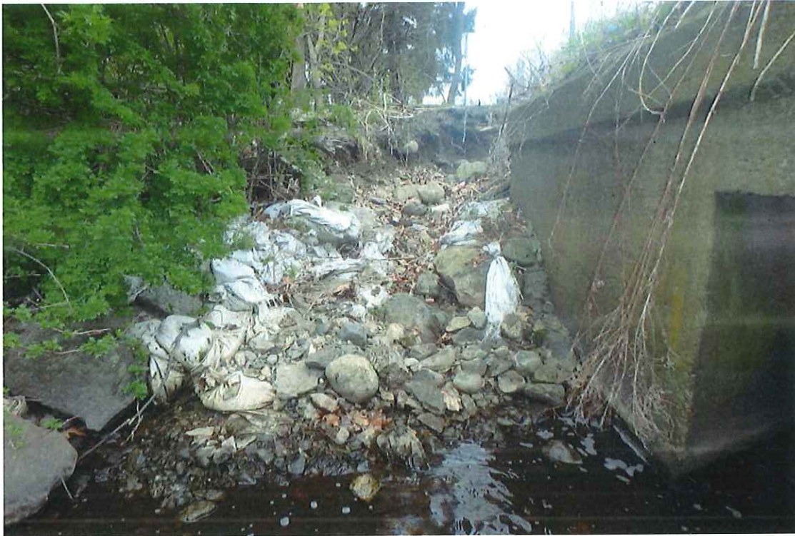
Photo 21: Northeast slope: Failed slope protection repair.
