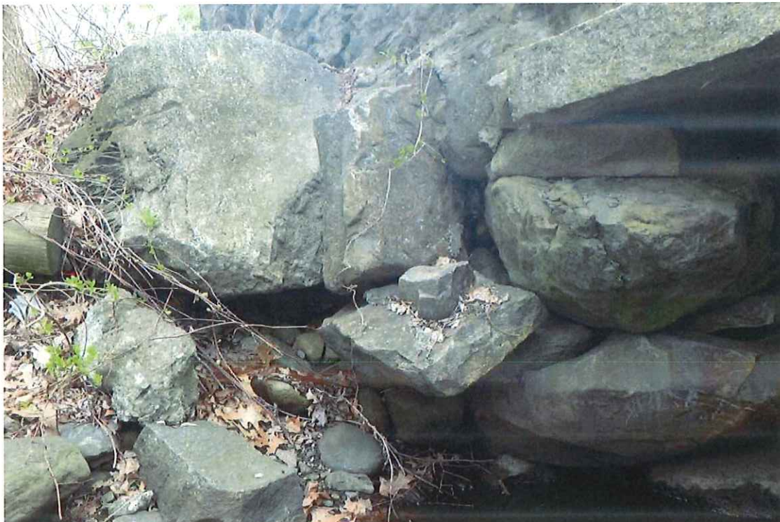
Photo 20: Southwest wingwall: Collapsed.
