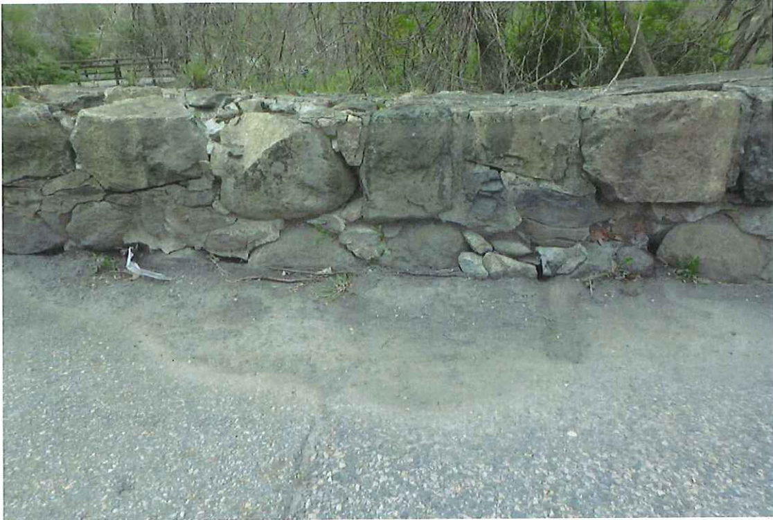
Photo 5: South masonry stone wall: Cracked mortar and missing pointing between the stones leading to water intrusion. South Sidewalk: Depression along masonry wall.
