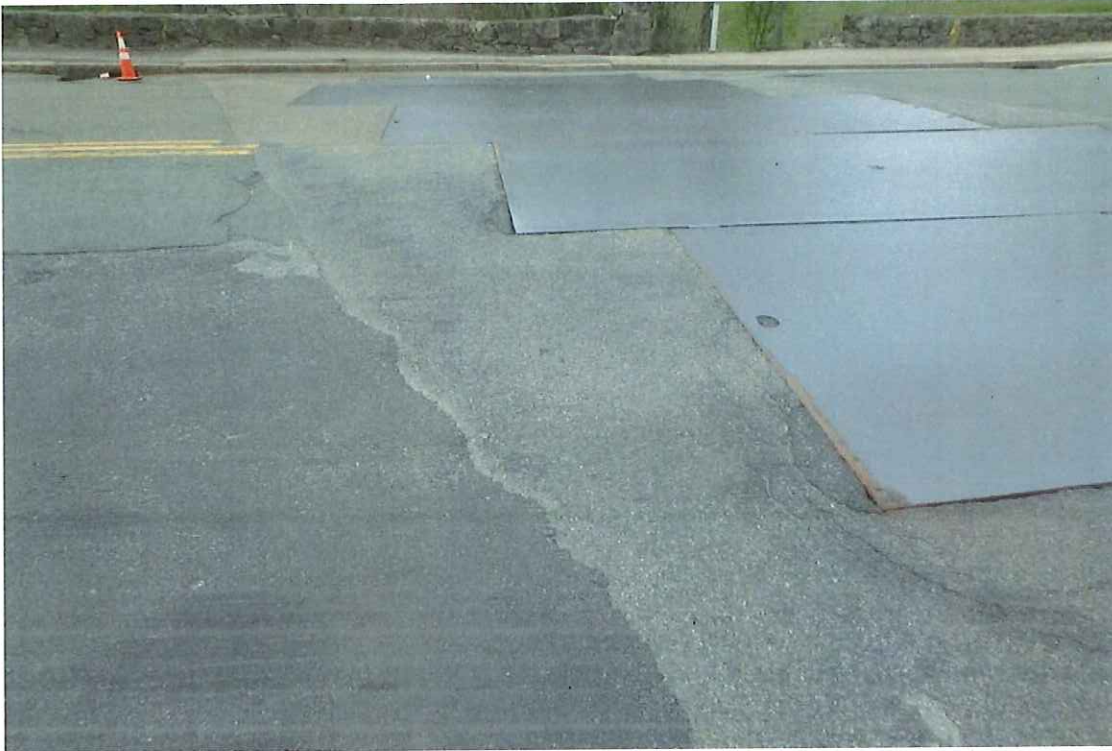
Photo 3: Steel Plate 4 and 5 at the northeast corner repaired potholes and a 2'-0" W x 7" L patch with radial cracking.
