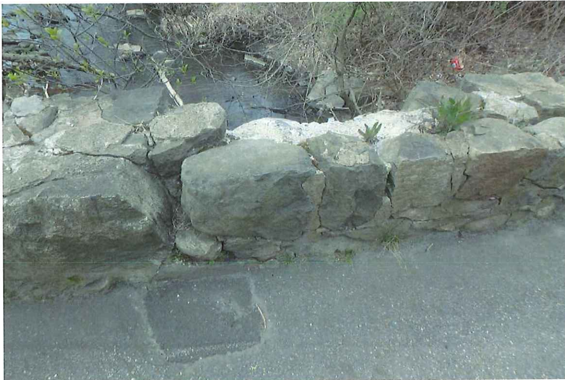
Photo 4: Repaired hole in south sidewalk. Missing stones and mortar in south railing.
