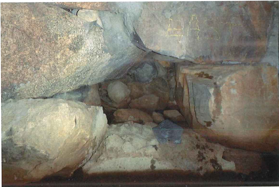
Photo 18: East breastwall: Void in first course of stone above waterline under slab 5.
