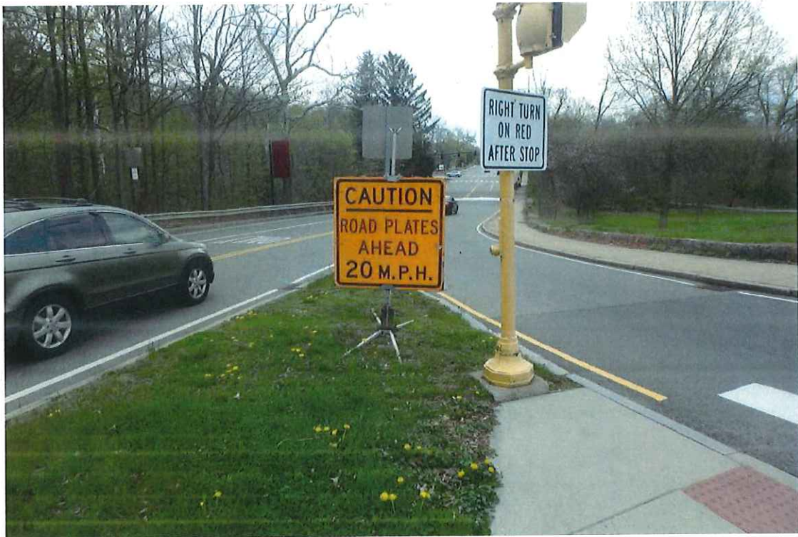
Photo 1: "Caution" sign in-place at the west approach.
