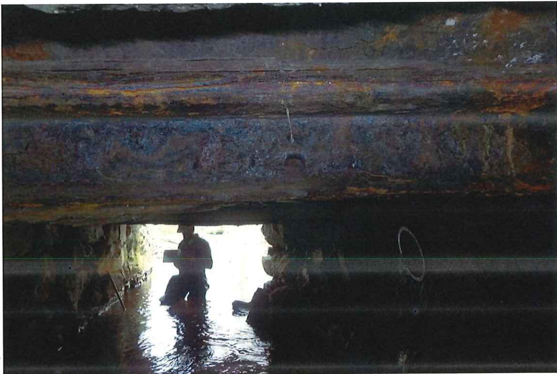
Photo 14: Steel beam 8: Severe section loss at the bottom flange up to 2.5' long x up to 2" wide.
