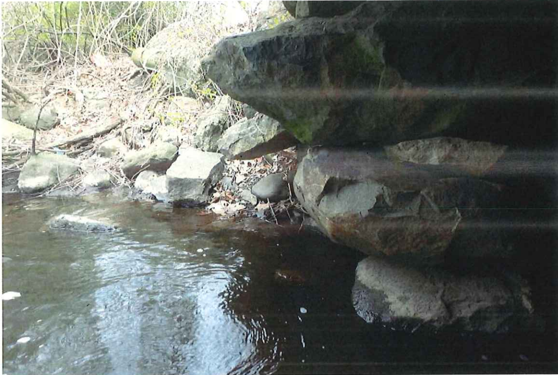
Photo 15: West breastwall: Large voids and missing stones at the south end.
