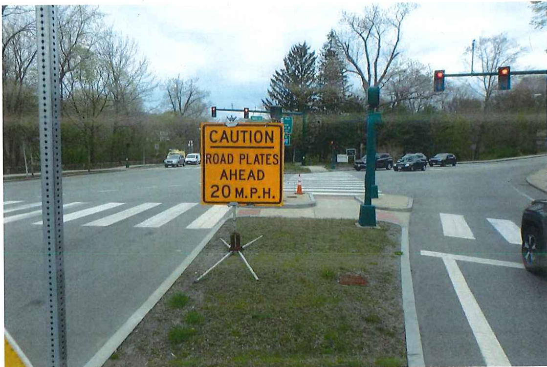
Photo 2: "Caution" sign in-place at the east approach.
