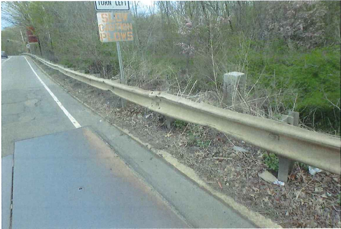
Photo 7: North bridge rail: Impact damage.
