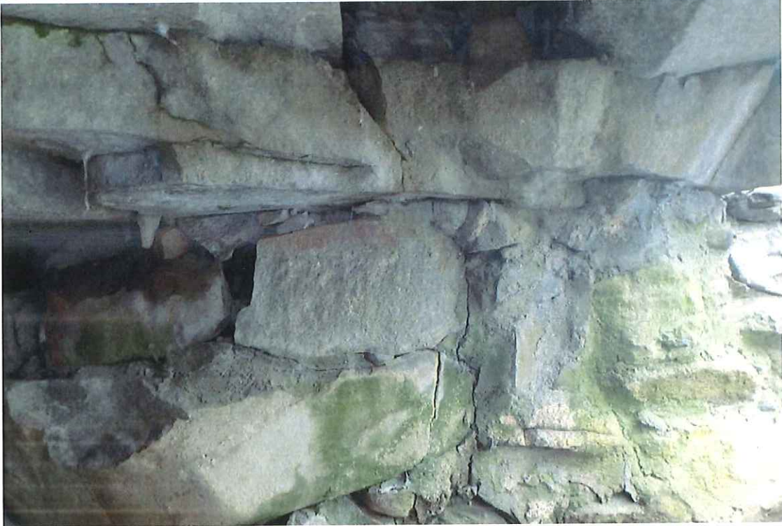
Photo 17: East breastwall: There are multiple stones with vertical cracks at the south end below beam 1.
