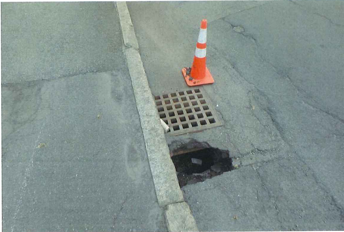
Photo 9: East approach: Sinkhole next to catch basin.
