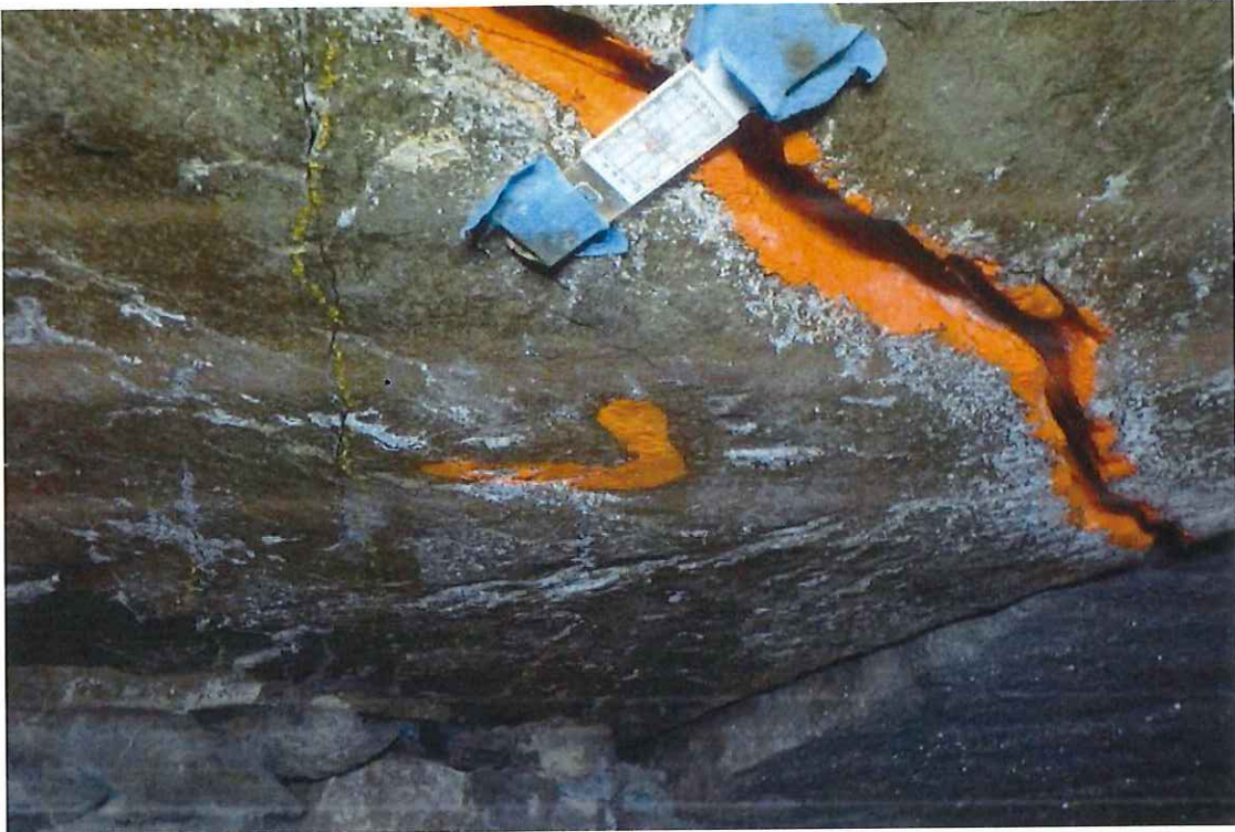
Photo 11: Granite slab 7: Transverse split up to 2" wide near midspan.
