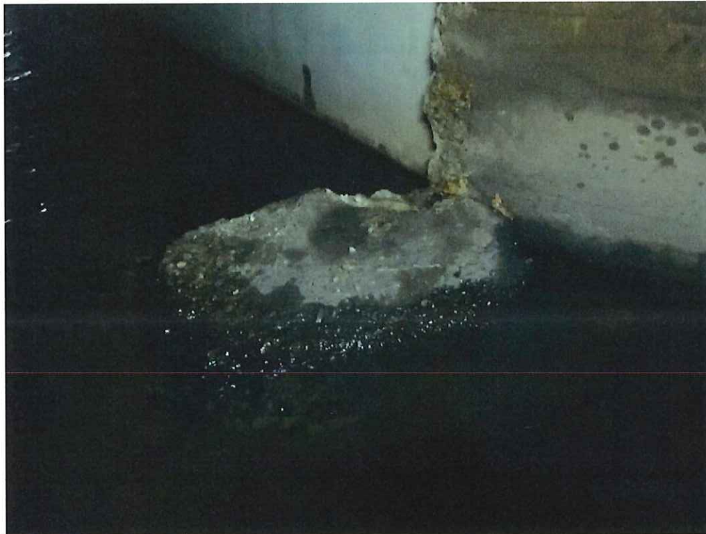
Photo 6: Floor, northeast corner, there is a 3' wide x 2.5' mass of concrete cast onto the floor.
