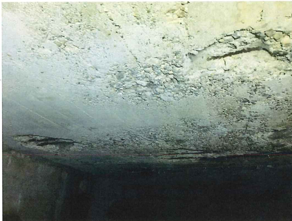
Photo 2: Station (00+18) to Station (00+30), 12' L x full width area of delamination, heavy scaling and multiple spalls, up to 3' L x 4'-8" W x 1.5" D with exposed and rusted rebar.
