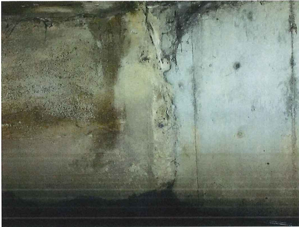
Photo 7: West wall, north fascia, full height x full width x up to 11" D spall with exposed and rusted rebar.
