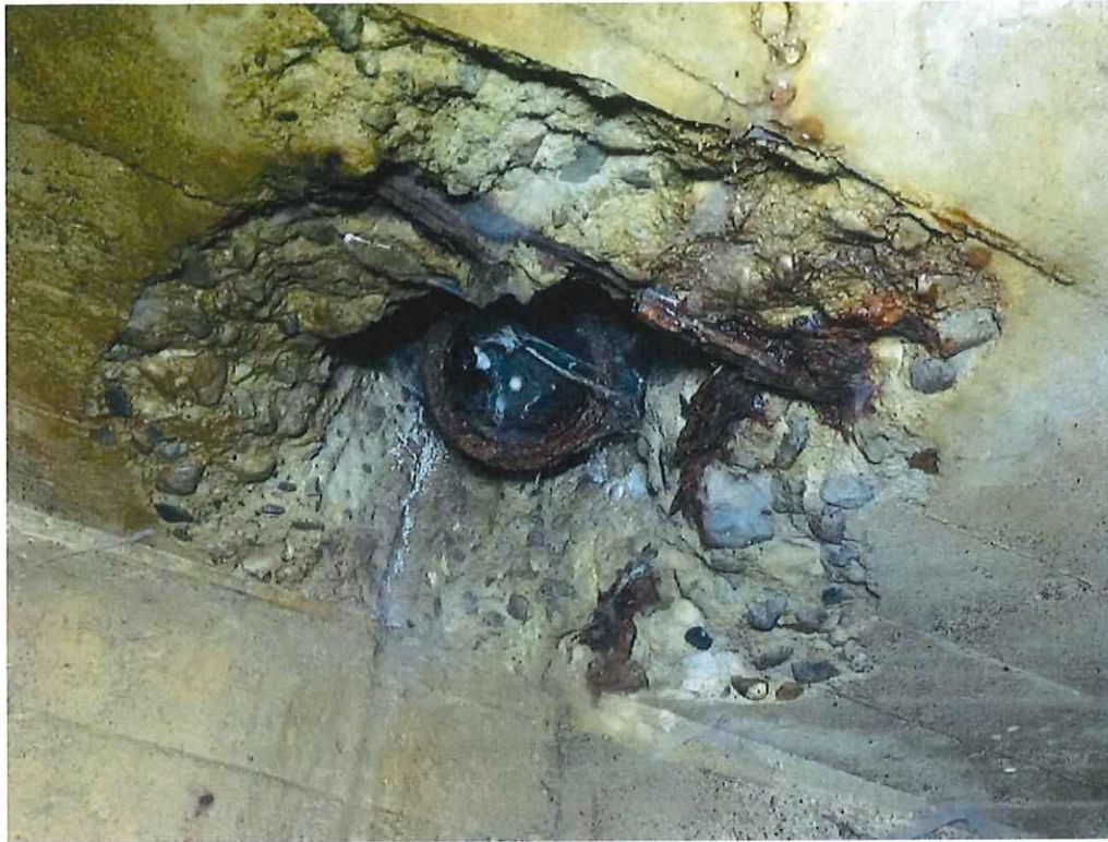
Photo 5: Station (00+47), 2'-2" L x 22" W x 11" D spall with exposed and rusted rebars with 100% section loss around the utility pipe.
