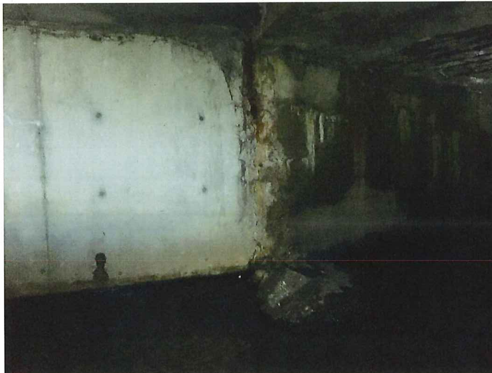
Photo 12: East wall, north end, full H x full width x 7" D spall with exposed and rusted rebar.
