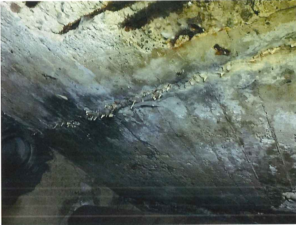
Photo 3: Station (00+25), active leakage at the construction joint with heavy efflorescence and rust staining.
