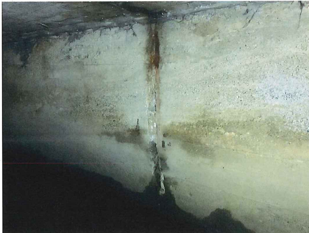
Photo 8: West wall, Station (00+06), full height x 4" W x 2.5" D spall, heavy rust staining and a full height x 1/8" W crack that extends into the roof with light efflorescence.
