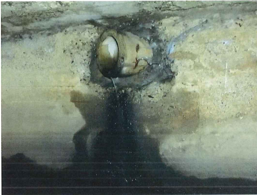
Photo 9: West wall, Station (00+17) around the 12" diameter RCP, 2.5' H x 3.5' L x 2.5" D area of scaling.
