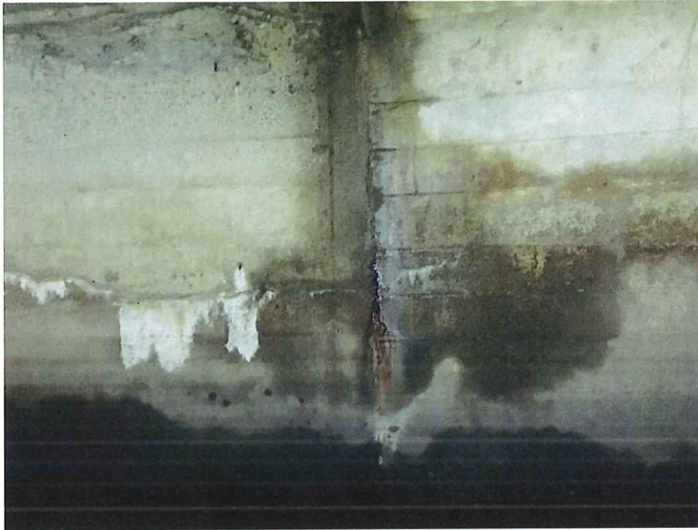
Photo 15: East wall, Station (00+47) at the construction joint, area of rust staining and active water leakage with light efflorescence.
