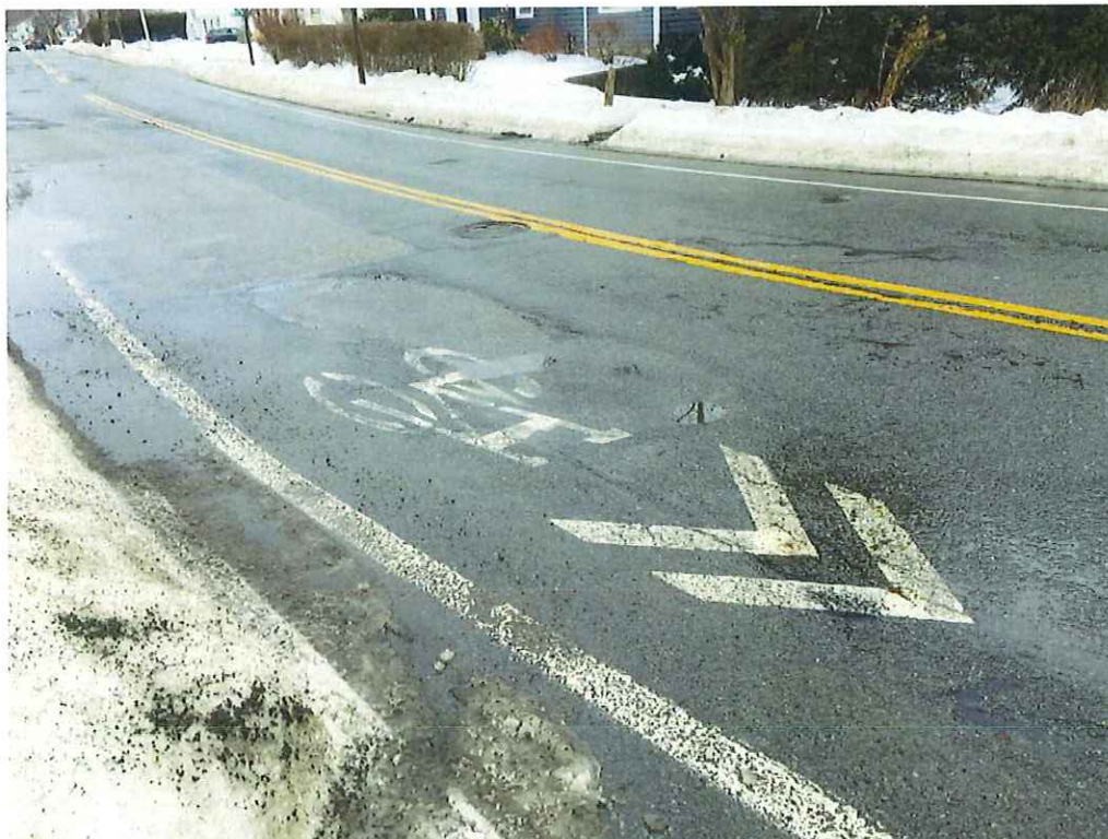
Photo 16: Eastbound lane, minor depression and a 7' L x 2.5' W patch.
