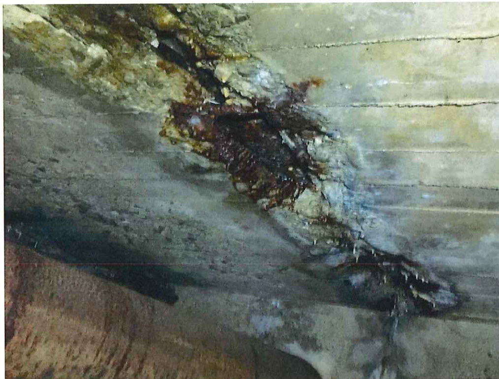
Photo 4: Station (00+31), 2.5' L x full width x 4" D spall with exposed and rusted rebars in both direction. There is heavy rust staining and active leakage around the incased steel pipe inside the roof.
