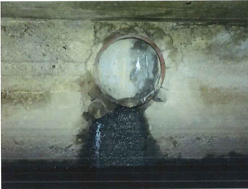
Photo 11: West wall, Station (00+40) below the 24" diameter utility, 2'-3" H x 20" W x 5" D area of scaling and active leakage.
