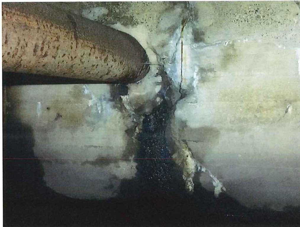
Photo 14: East wall, Station (00+32) below steel utility pipe, 2.5' H x 2' W x up to 3" D area of heavy scaling and water leakage. Also note the full height vertical crack with heavy efflorescence.
