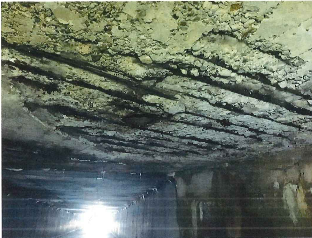
Photo 1: Station (00+08) to Station (00+14), 6'-3" long x full width x 2.5" deep area of spalling with exposed, rusted rebar and up to 100% section loss.
