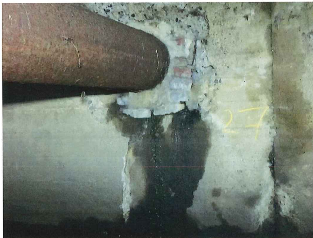
Photo 10: West wall, Station (00+27) around the steel utility pipe, 2'-4" H x 2'-8" W x 3" D scaling with active leakage and 2' long vertical hairline crack with efflorescence.
