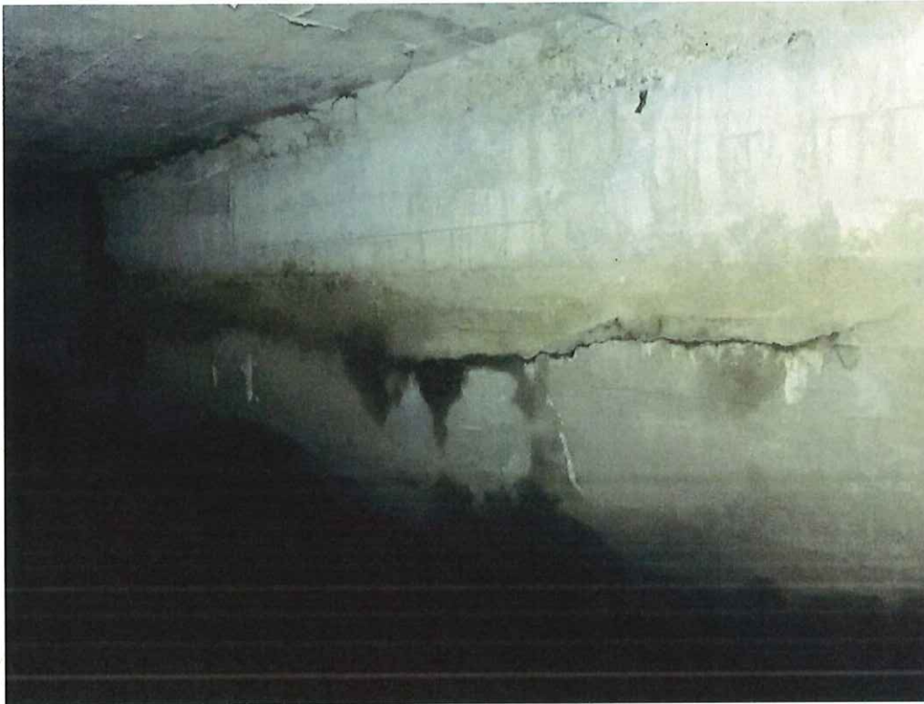
Photo 13: East wall, full length, 1/8" wide horizontal crack with areas of efflorescence and water staining.
