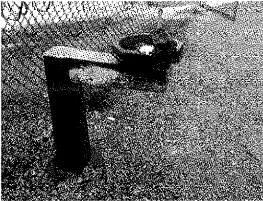
Water fountain rusted and not working. Should be removed.
