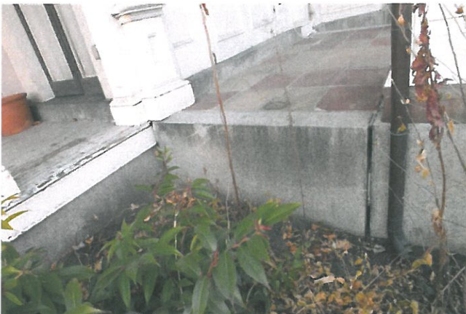
11. Paving at front porch has settled.
