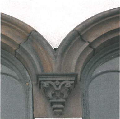
Open joints at stone window arches
