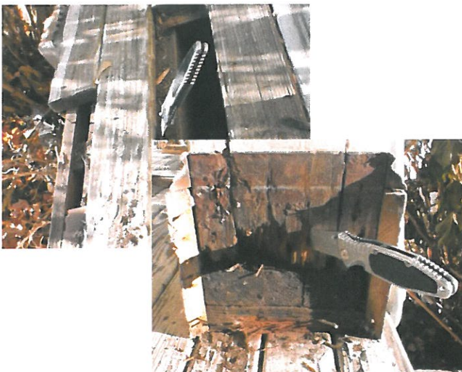
17. Rot in east piazza joist in upper photo. Rot in column base at east piazza lower photo.
