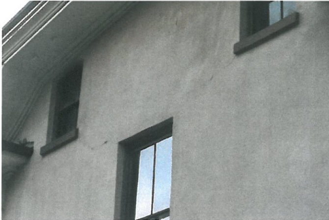
18. Cracks in stucco at second floor. These are new since 1995 painting.
