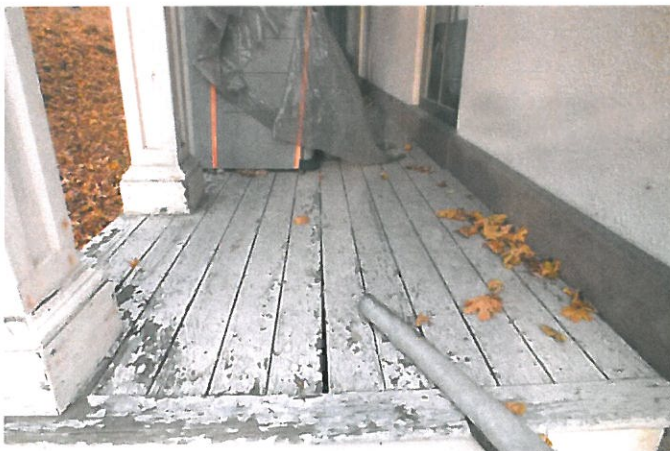
5. Rear piazza deteriorated deck condition.
