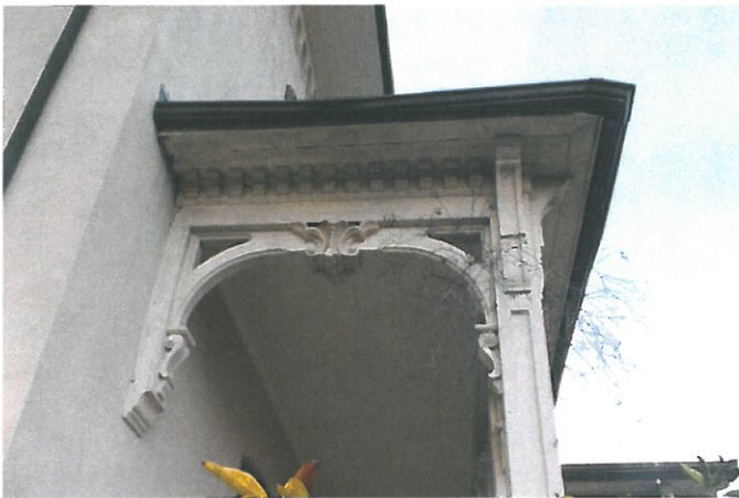
10. Roof bracket at front west piazza may have pulled slightly from building.
