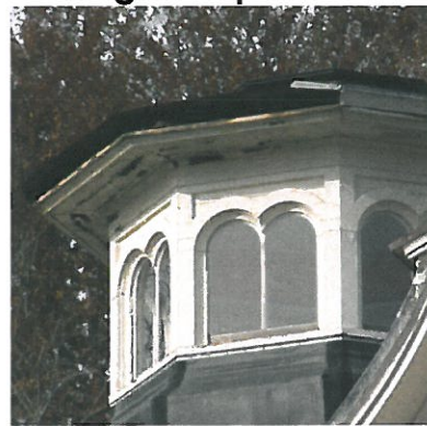
Damaged cupola roof
