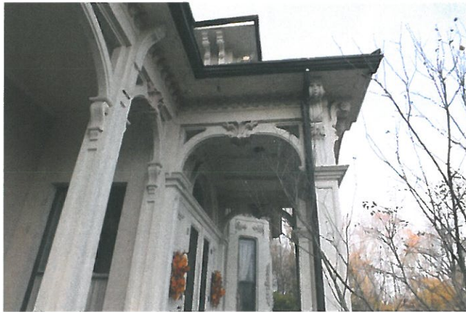
13. Roof over porch has settled along with settlement of porch landing. Columns moved with foundation to out of plumb position.
