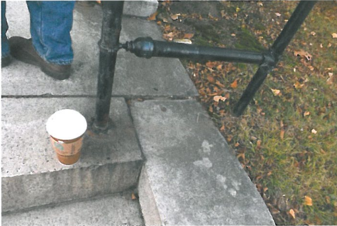
15. Cheek walls to front stairs have settled. East cheek in foreground.
