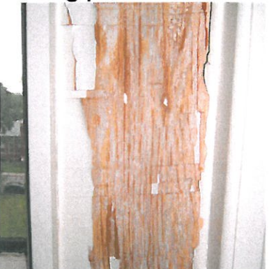
Peeling paint due to moisture
