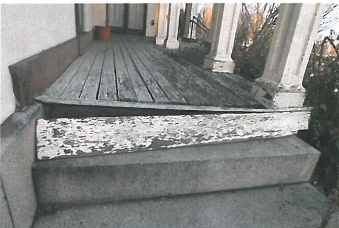
8. Front west piazza deteriorated deck condition.
