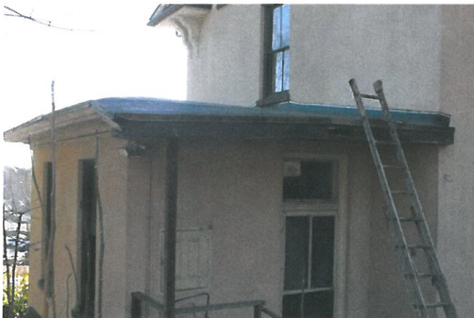
20. Access setup to review opening at edge of roof over ice chest entry.
