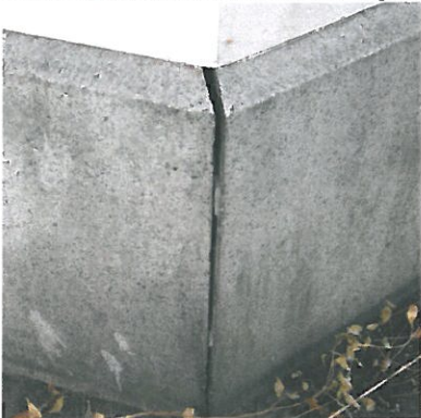
Deteriorated mortar; open joints at foundation
