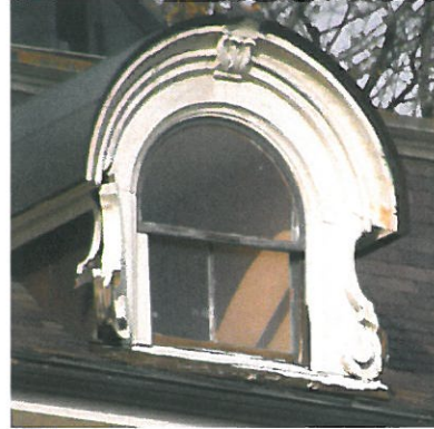
Broken and damaged scrolls
