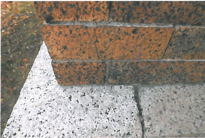
7. Cracks in brick in west chimney where granite foundation facing has opened up at head joint.
