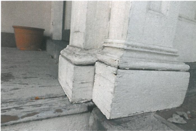
12. Old repairs to column bases disregard alignment at bases.
