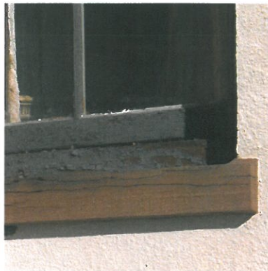
Split brownstone sill and peeling paint
