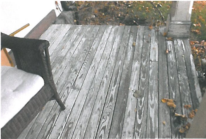
16. Decking at front east piazza is worn.
