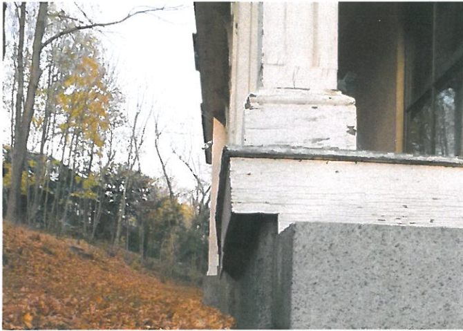
6. Dislocated foundation at rear piazza.
