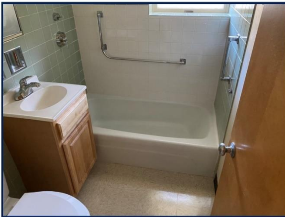
Most bathroom fixtures are original to 1970s, and some bathrooms have water damage
