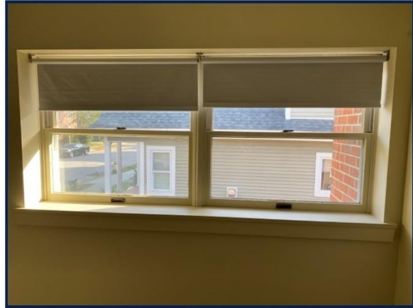
Single-pane, uninsulated windows are not energy efficient. Given their age, replacement parts are not available, making it difficult to maintain them in operable condition
