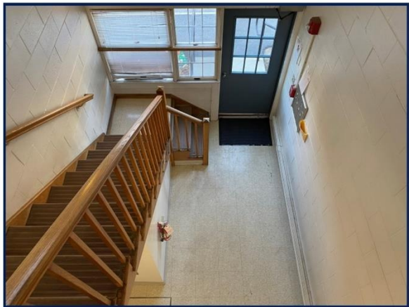
Second-floor units require use of a steep and narrow staircase
