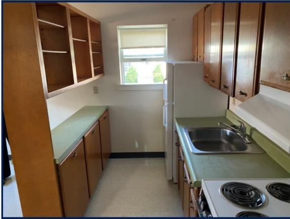
Kitchens are original to the 1970s, with finishes in worn condition and some kitchens showing signs of water damage. Stoves are not full size and there is inadequate food preparation area
