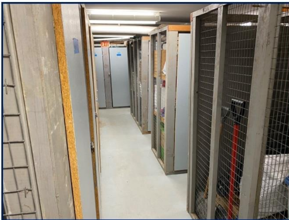
Resident storage is located in basement of community building and prone to flooding
