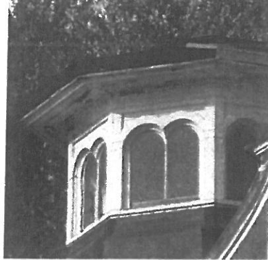
Damaged cupola roof
