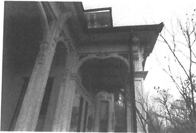
13. Roof over porch has settled along with settlement of porch landing. Columns moved with foundation to out of plumb position.
