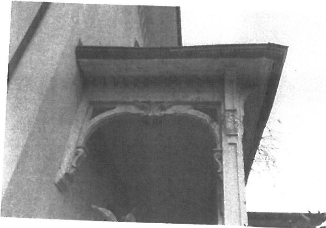
10. Roof bracket at front west piazza may have pulled slightly from building.
