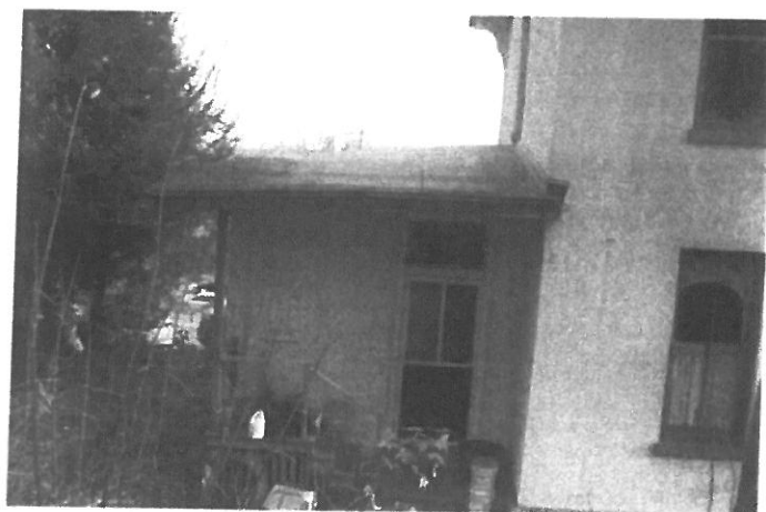
4. Ice chest stairs and roof extension framing materials not in historic context.
