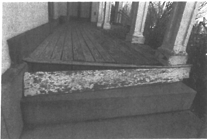
8. Front west piazza deteriorated deck condition.
