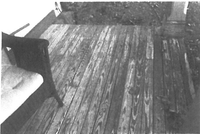
16. Decking at front east piazza is worn.
