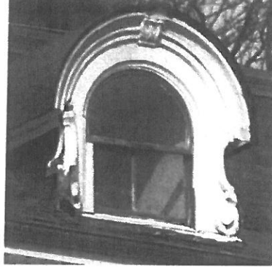
Broken and damaged scrolls
