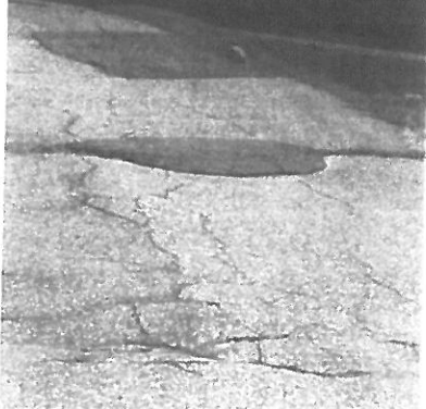
Drive cracking and patching
