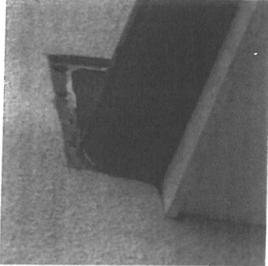
Exposed stucco at roof intersections
