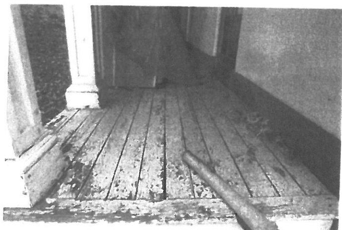
5. Rear piazza deteriorated deck condition.
