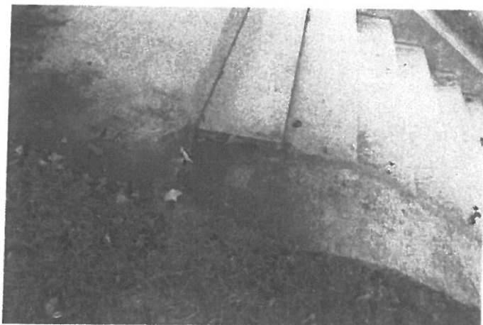
14. Cheek walls to front stairs have settled. West cheek in foreground.
