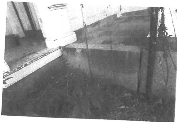
11. Paving at front porch has settled.
