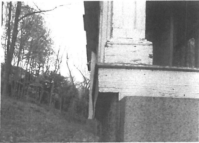
6. Dislocated foundation at rear piazza.
