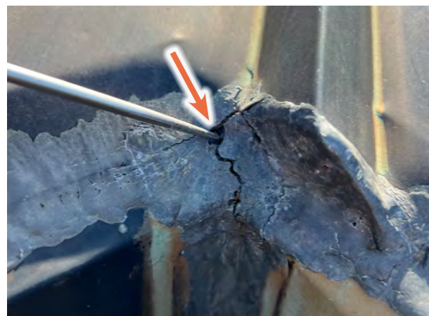
Image C-25: Large cracks at the intersection of copper valleys and gutters allow considerable water to enter and rot the woodwork.
