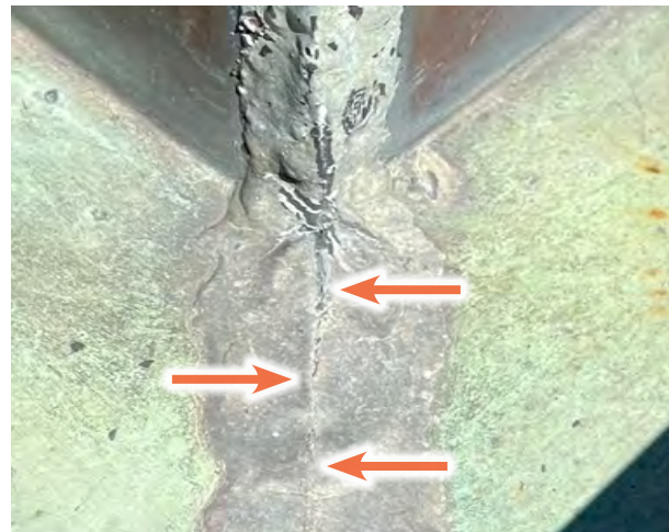
Image C-24: Hairline cracks at gutter miters suggest poor/inconsistent solder penetration.
