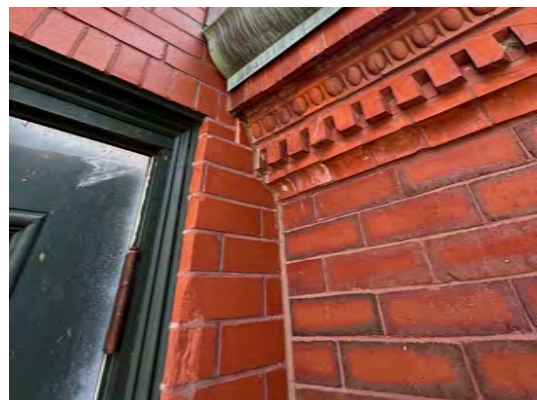
Image A-42: Spalling and deterioration of the masonry opening around the door to the fire escape.
