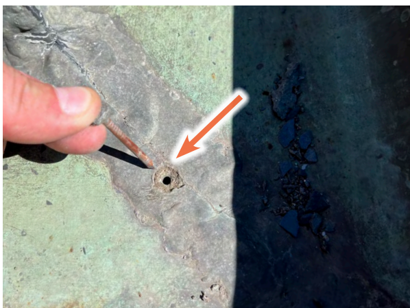
Image C-22: Nail holes in the solder joints render them virtually useless.
