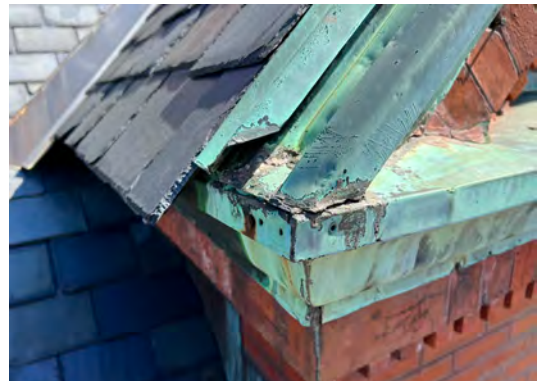
Image A-10: View of deteriorated decorative copper moldings at the south gable end. Condition is typical across
