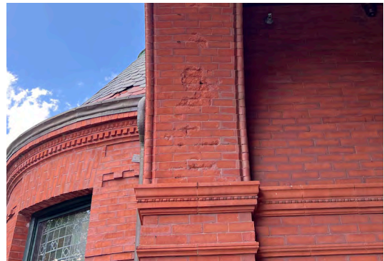
Image A-25: Isolated spalling at the west side of the intrados of the main entry arch.
