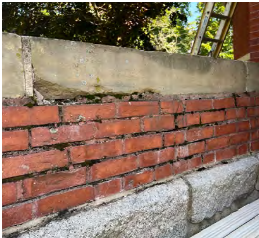
Image B-27: Severely deteriorated south site wall caused by water infiltration through sky-facing joints.
