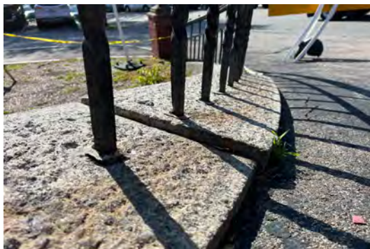
Image A-58: Original metal handrails embedded in the granite coping stones at the south retaining wall.
