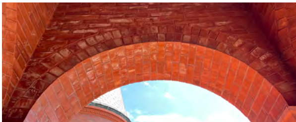
Image A-27: Area of efflorescence at interior brick masonry above east facing arch of south portico.
