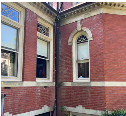
Image B-21: Severe brick masonry and mortar deterioration caused by ineffective copper gutters and downspouts.
