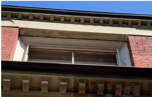
Image B-26: Bulging lintel at top floor or east projecting
