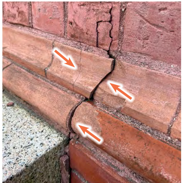
Image C-57: Upward thrust of the rotating granite cheek walls have cracked the brickwork at the intersection, consistently.
