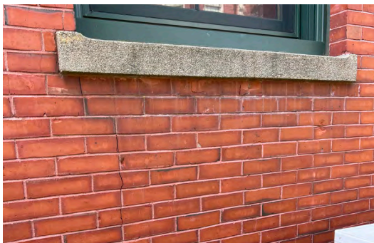
Image A-37: Vertical cracks in brick masonry below the first floor cast stone window sills at the north elevation.
