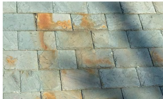
Image B-03: Oxidized slates at original slate roof on School Administration Building.
