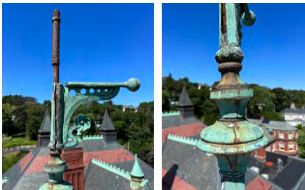
Image A-14: Significantly deteriorated original copper weathervane at the top of the turret. Much of the weathervane is missing.
