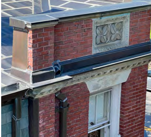
Image B-20: Through-parapet drainage detail suspected of compromising/damaging brick and sandstone masonry.
