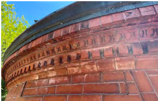
Image A-29: Mortar deterioration and efflorescence at decorative brick cornice caused by prior leaking gutters.
