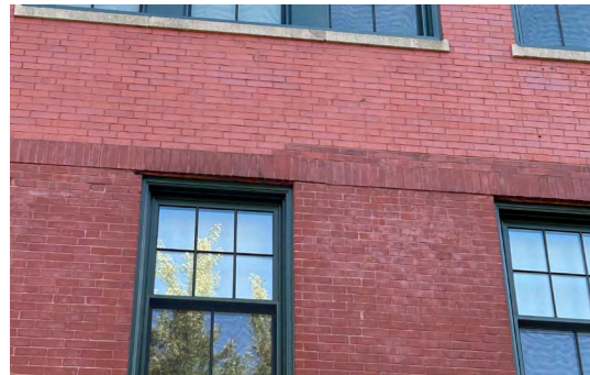
Image A-39: Area of bulging brick masonry at second floor window at north elevation due to rust jacking.
