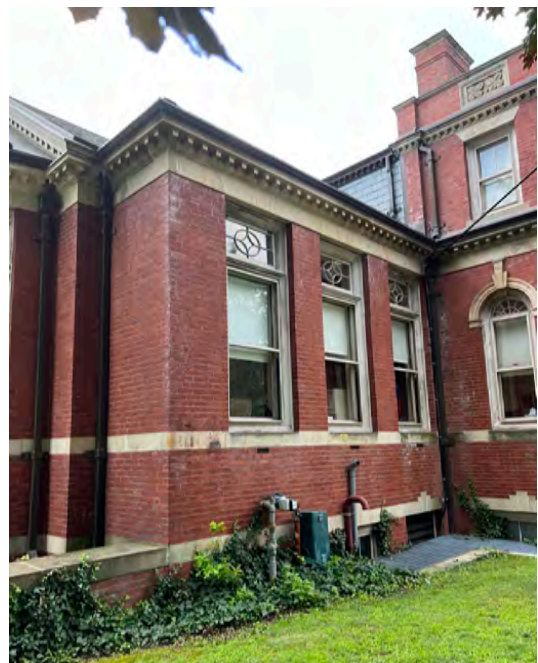
Image B-18: View of northwest corner of the building showing deterioration to sandstone cornice and brick masonry.
