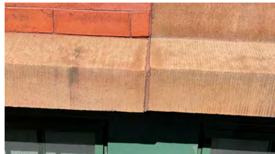
Image A-40: Movement at the modified brownstone lintel at the south elevation due to rust jacking
