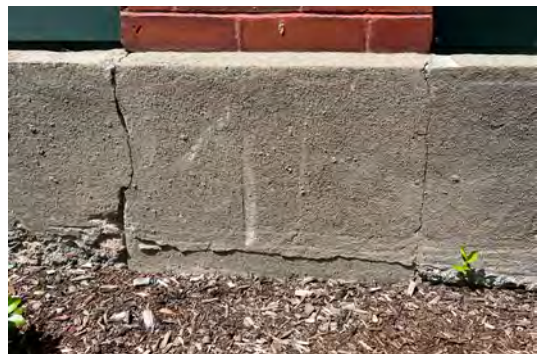
Image A-62: Cracks in the parge coat at the concrete foundation where the bay doors were infilled.
