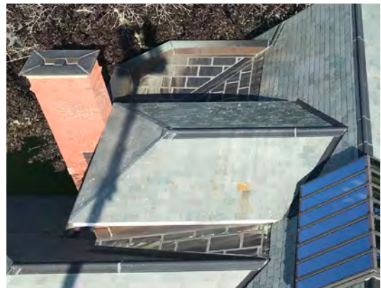
Image B-10: Roof of elevator override directly abutts south chimney focusing water and snow on rear chimney wall.
