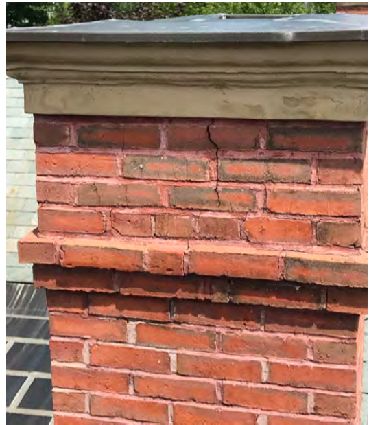
Image B-12: Significant structural cracking at the top of the south chimney. Note the deteriorated capstone.
