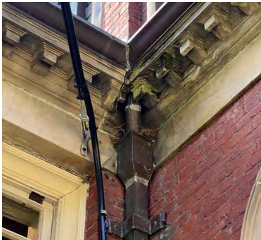
Image B-19: Blocked collector box at downspout causing significant damage to sandstone cornice and brick masonry.
