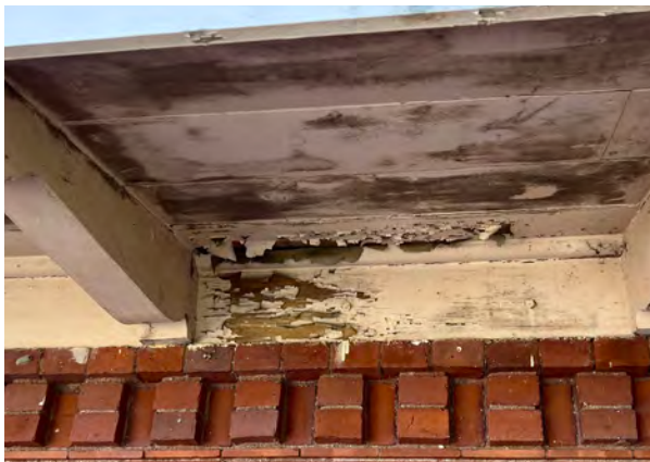
Image C-35: Flaking paint is prevalent at sites where water has entered the cornice and framing.
