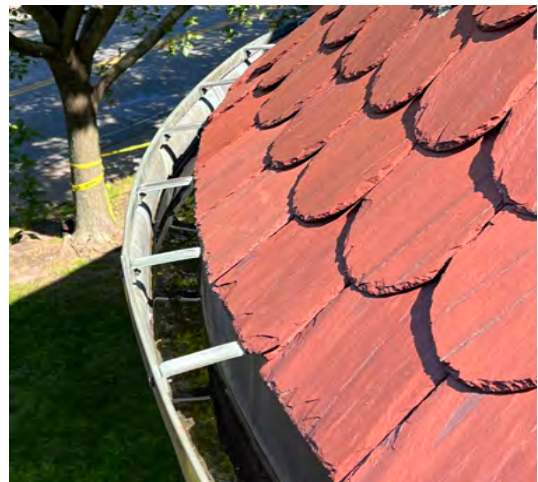
Image A-19: Water and debris collecting in the gutters away from the downspouts, suggesting an issue with the pitch.
