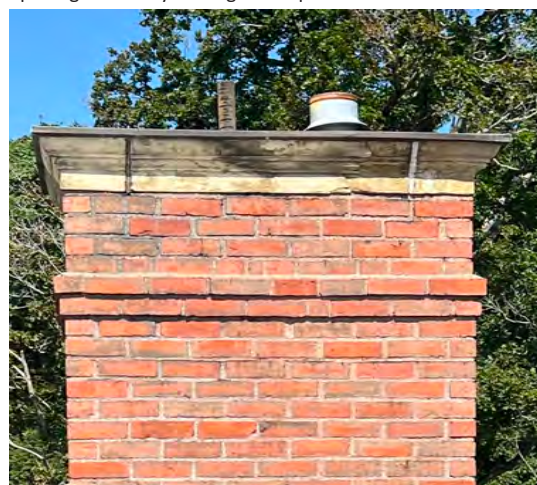
Image B-25: Deteriorated capstone at chimney.
