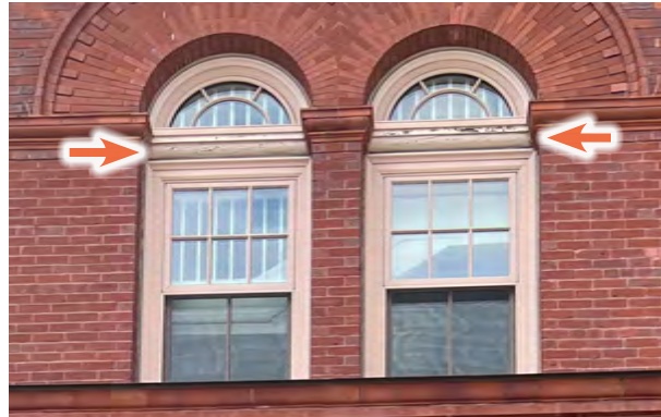
Image C-40: Two pairs of windows retain the sole visible woodwork, long since replacement by modern units.
