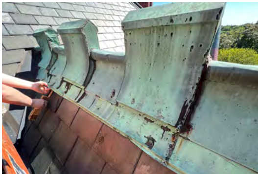
Image A-07: Ferrous nails were driven through the crestring to attach it to the roof. Mastic used to seal broken seams.
