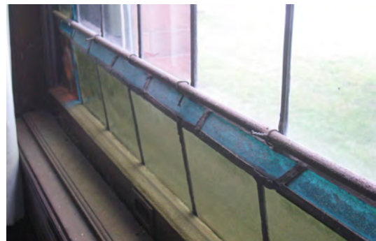
Image A-48: Buckling and deteriorated lead joints at large stained glass windows at the west elevation.
