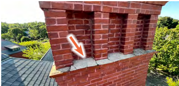
Image C-44: A deteriorating mortar wash at the chimney should be replaced to ward off standing water.
