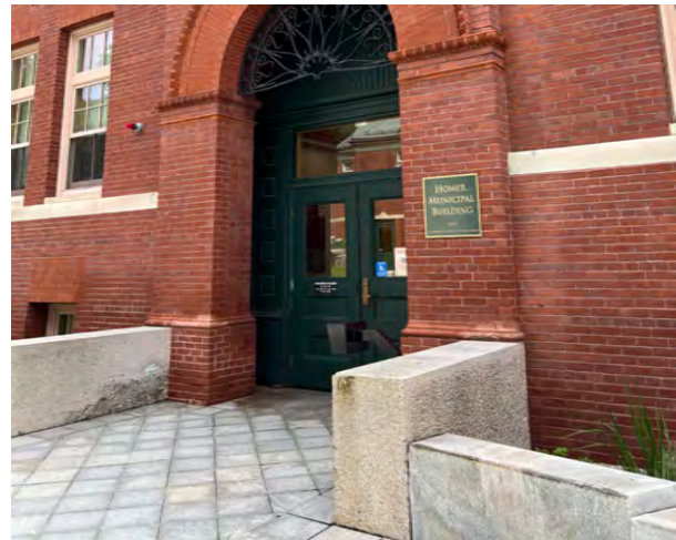
Image C-58: Similar rotating granite cheek walls have damaged the west entry brickwork as well..
