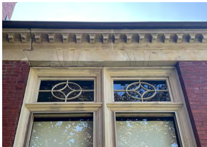
Image B-22: Deteriorated and cracked mortar joints at sandstone cornice caused by ineffective copper gutters and downspouts.
