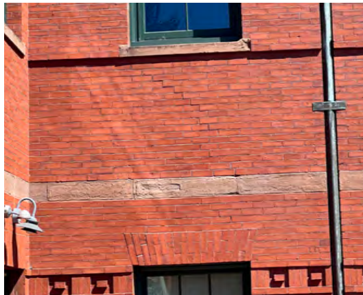
Image A-21: Slipping jack arch and step cracking at ground floor windows at south elevation
