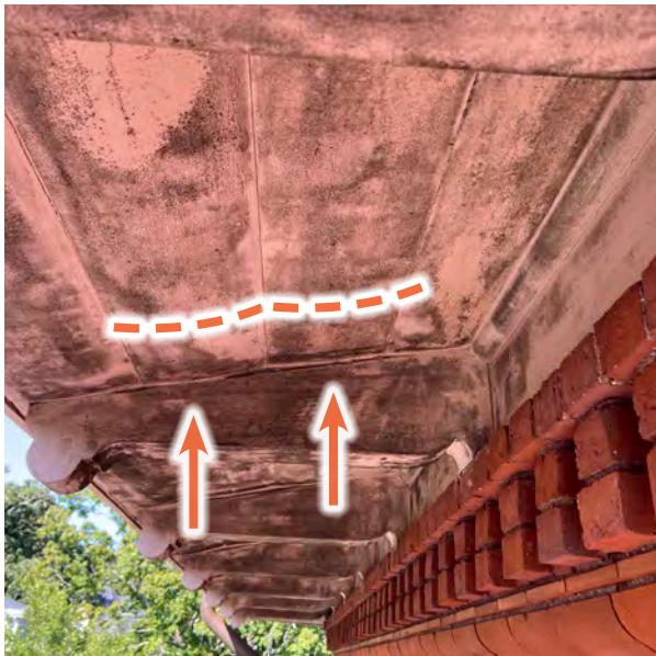
Image C-34: Cupping soffit boards suggest they have been damp in years past, possibly due to low-quality woods used in replacement..
