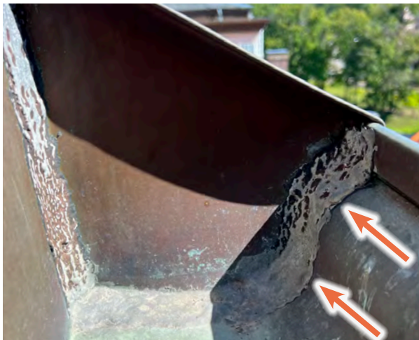
Image C-21: Hairline cracks at solder joints are a site for water to infiltrate the wood cornice below.
