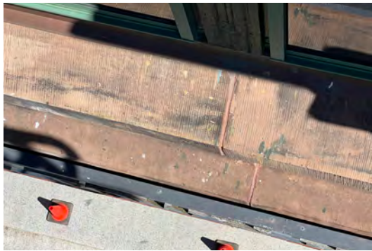
Image A-51: Sky-facing joints at large brownstone sills are susceptible to water infiltration and deterioration.
