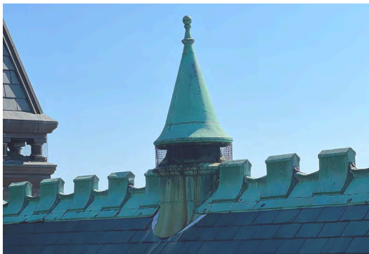
Image A-08: View of copper ventilation cupola intergrated with the crenelated crestring at the north-south ridge.
