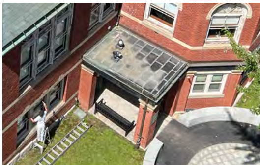
Image B-06: Flat seam copper roof over east portico. Evidence of ponding present around spotlights.
