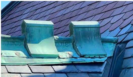
Image A-06: Original crenelated copper crestring is in poor condition due to age and weathering.
