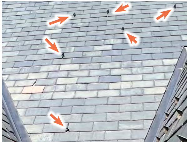
Image C-15: An inconsistent array pattern of snowguard pads suggest many had been ripped off by snow/ice.
