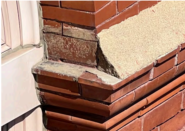
Image C-53: Although some in intact, chunks of the steep wash are randomly missing, mostly at the inner arch returns.
