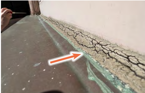
Image C-33: Cracked sealants between aluminum or vinyl windows and copper require replacement overall.
