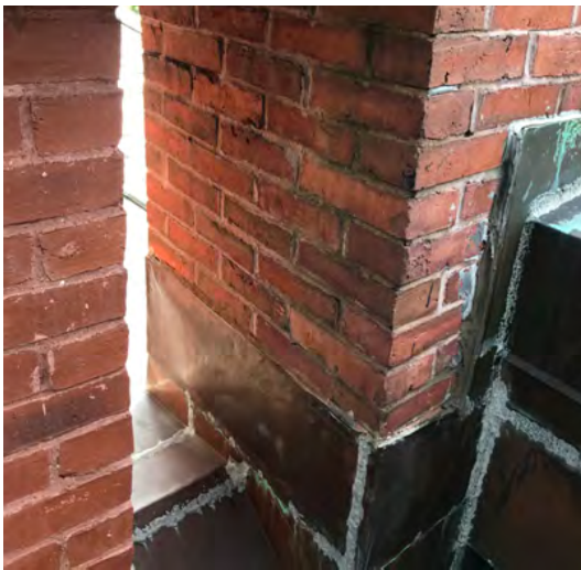
Image B-14: Poorly detailed copper counterflashing detail at chimney. No visible clips and new sealant joints required.
