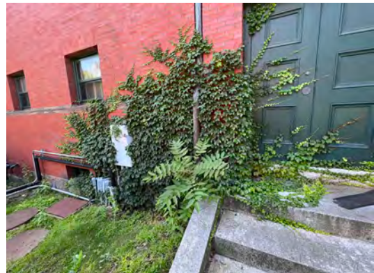
Image A-60: Vine overgrowth at brick masonry and granite stairs along the north elevation.
