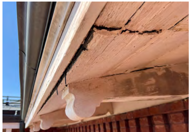
Image C-38: The worst of the woodwork is easily visible from below, requiring replacement.
