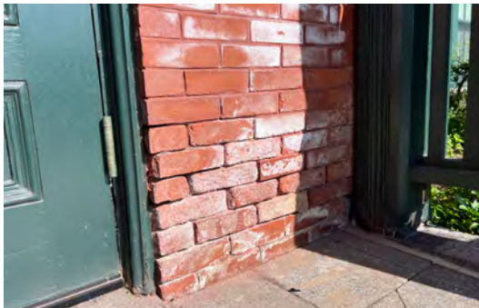
Image A-28: Deterioration and efflorescence at base of east entry vestibule caused by rising damp and de-icing salts.
