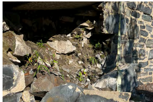
Image A-53: Dry-laid stone retaining wall backfilled with soil, no other structural support present.
