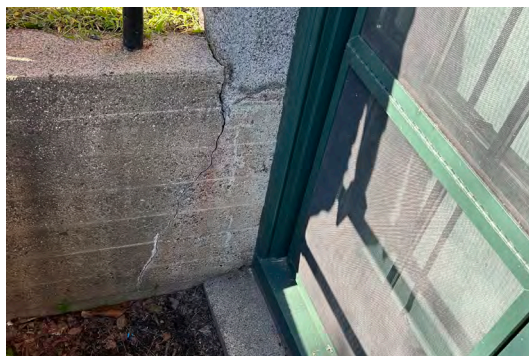
Image A-59: Crack at the concrete window well wall at the foundation on the south elevation.
