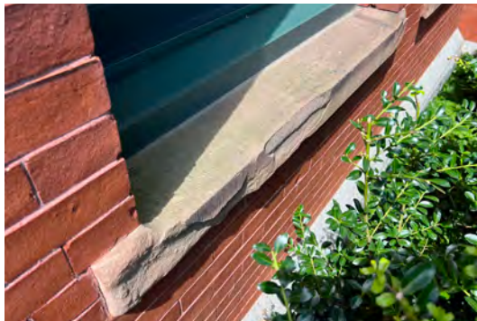
Image A-50: Cracking and spalling caused by the pressure of the load traveling down the edges of the masonry openings.
