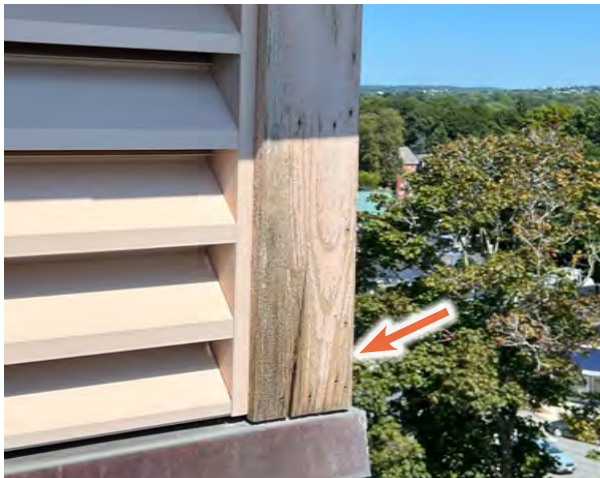
Image C-30: Low-quality wood corner boards have reached the end of their life.
