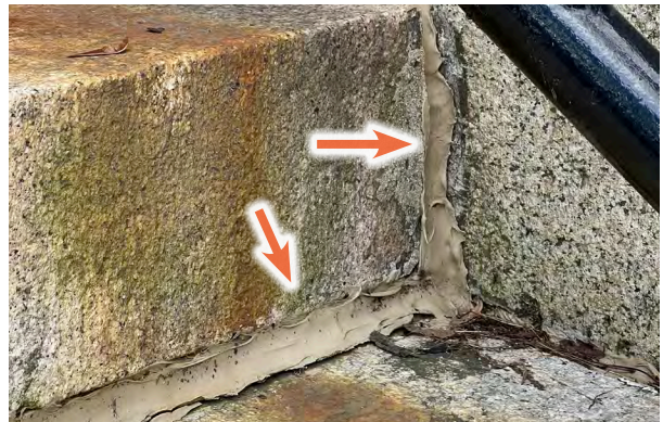
Image C-56: The slow shifting of granite treads are filled with sealants, wider and wider with each application.
