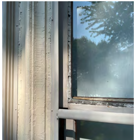
Image B-30: Close up of original window showing cracked glazing putty, aluminum storm window, and wood trim.
