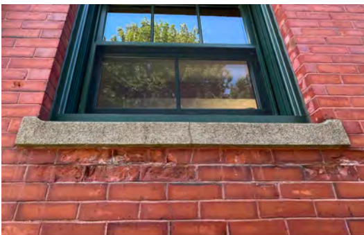
Image A-38: Spalling at brick masonry below the cracked first floor cast stone window sills at the north elevation.
