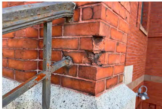
Image A-57: brick deterioration caused by twisting metal handrails as a result of the failing retaining wall.
