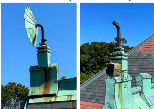
Image A-09: View of the original copper floral finial at the west gable end (Left) and the missing finial (Right)
