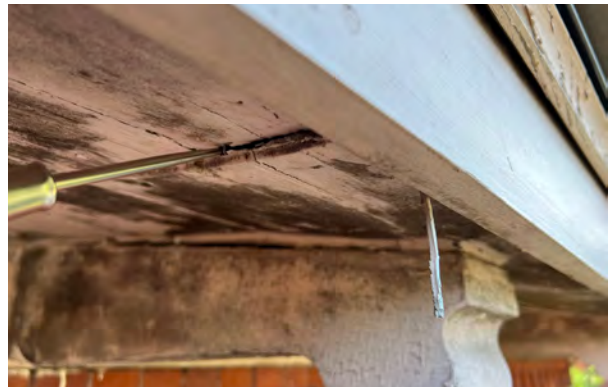
Image C-37: Soft end grain at soffit boards are pierced easily by an awl, suggesting they have been damp for some time.
