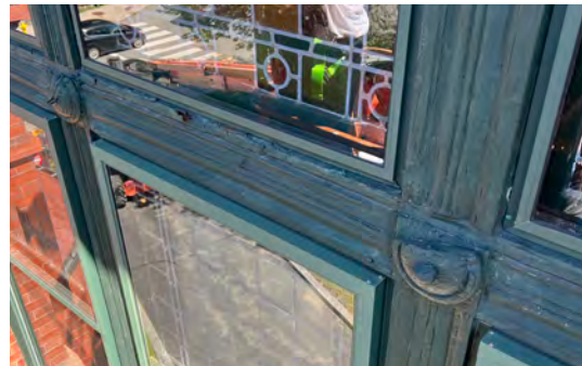
Image A-47: View of the deteriorated wood trim and bullseye rosettes at the south gable end's stained glass
