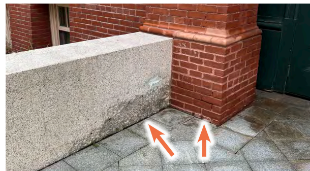
Image C-59: Excessive salts and de-icers at the high-traffic pavers have likely damaged both brick and granite.
