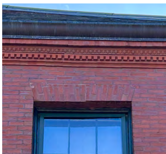
Image A-23: Slipping jack arch and step cracking at the second floor window at north elevation .
