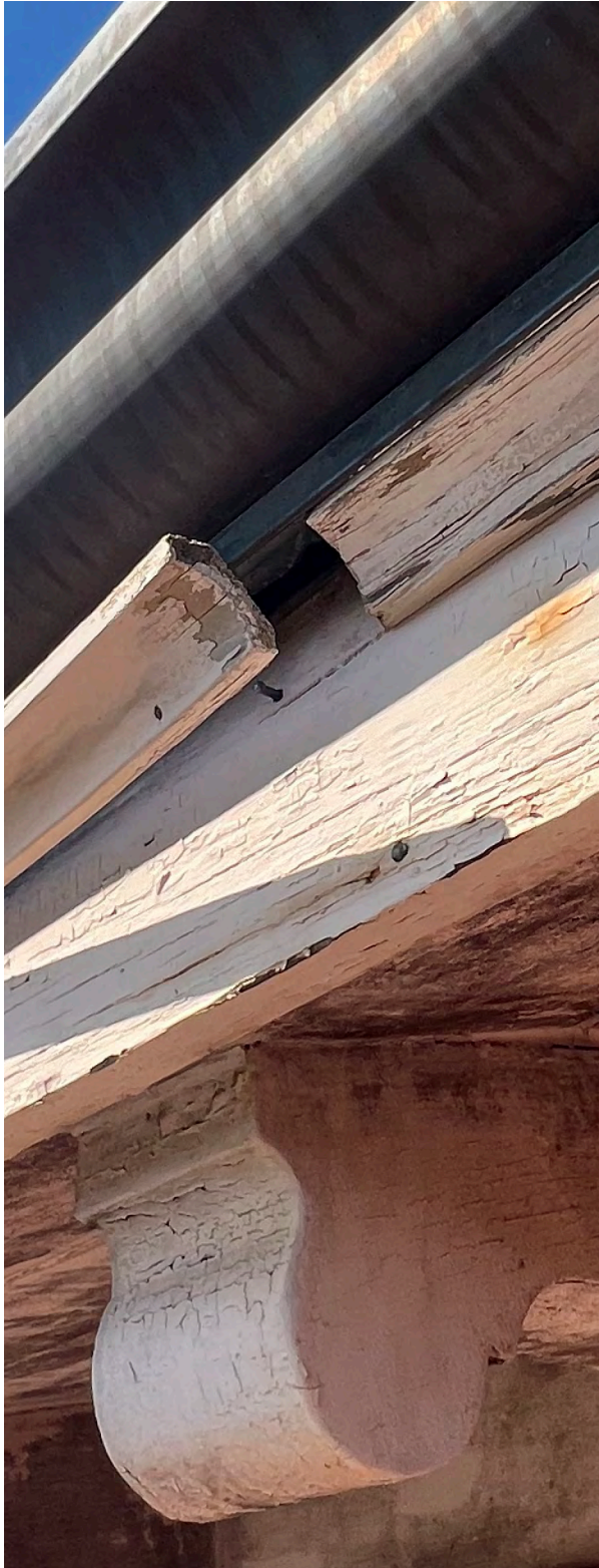
Image C-39: Thin and inexpensive bedmoulds for the gutters have not stood the test of time since gutter installation.
