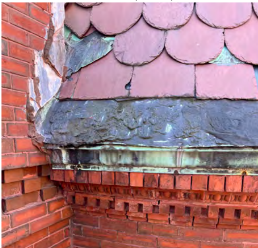
Image A-17: Severely deteriorated copper skirt, cornice, and flashing turret roof and chimney.
