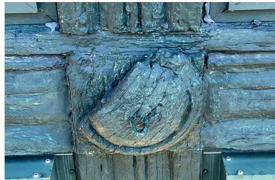
Image A-46: View of the deteriorated wood trim and bullseye rosettes at the south gable end's stained glass
