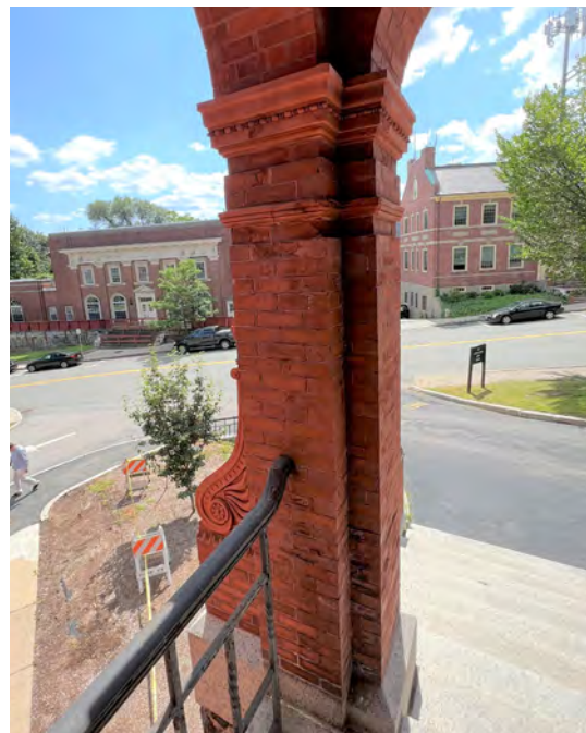
Image A-26: Deteriorated and spalling brick masonry at the interior of support column at south portico.
