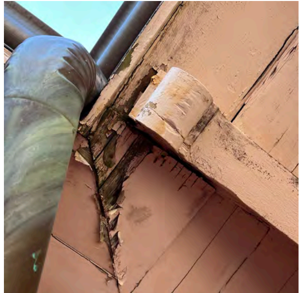
Image C-36: The worst of the cornice damage occurred at the inside corners of gutters where water is unimpeded.
