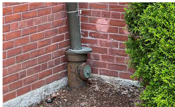
Image C-28: Cast iron boots collect rainwater, and divert it presumably into a subsurface storm water system.
