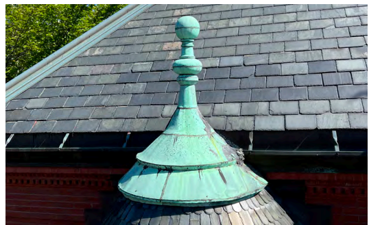
Image A-12: View of severely deteriorated original copper finial at south projecting bay window.
