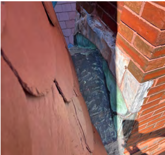
Image A-16: Deteriorated copper cricket and flashing between the turret and chimney. Heavily coated with mastic.
