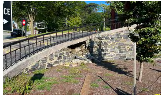
Image A-52: Collapsing retaining wall between the driveway and the courtyard at the southeast corner of the building.
