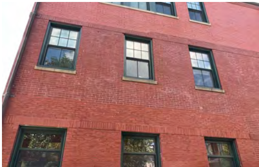
Image A-35: View of the north elevation of the Town Hall addition showing the three different brick colors.
