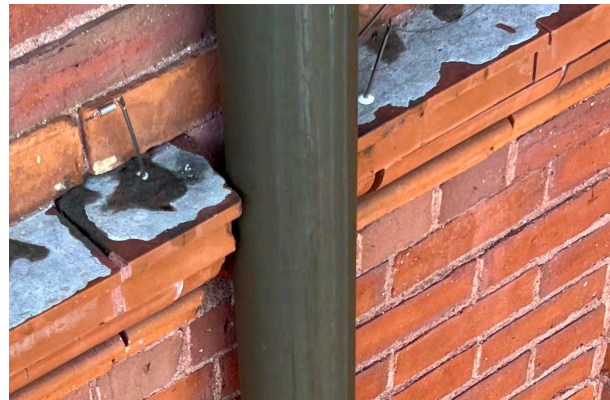
Image C-27: Copper downspouts are in good shape and their back-side seams appear intact and un-compromised.
