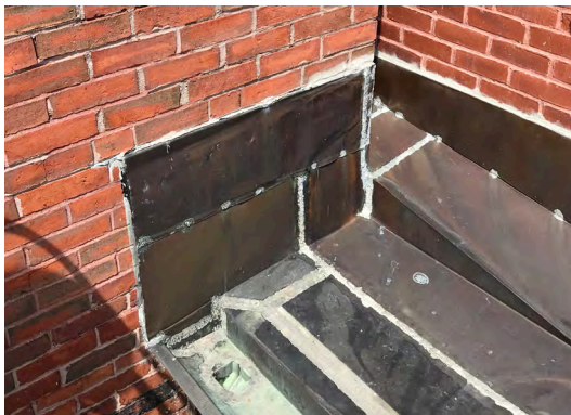
Image B-15: Poorly detailed copper counterflashing detail at chimney. No visible clips and new sealant joints required.
