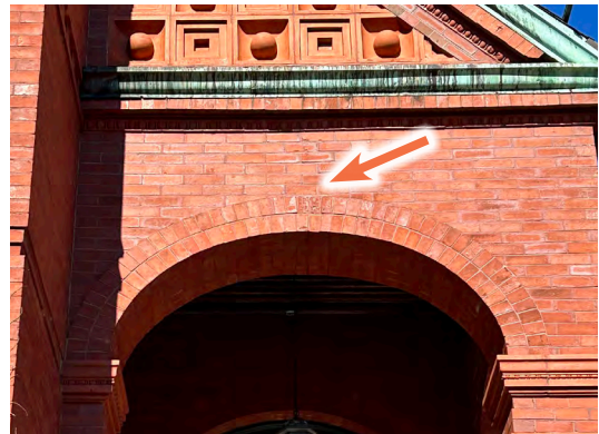
Image A-24: Slipping round arch and step cracking at the south portico. Note the broken keystone at the center of the
