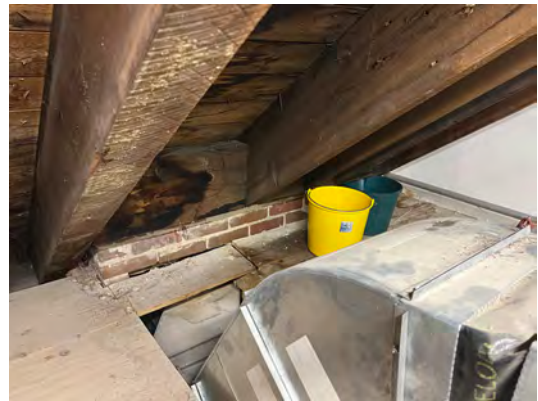
Image B-09: Interior leaks at attic level of School Admin Building. Buckets are used to capture leaks.
