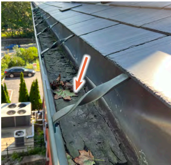
Image C-19: Compact gutter sediment and debris suggest improper pitch, allowing collection over time.
