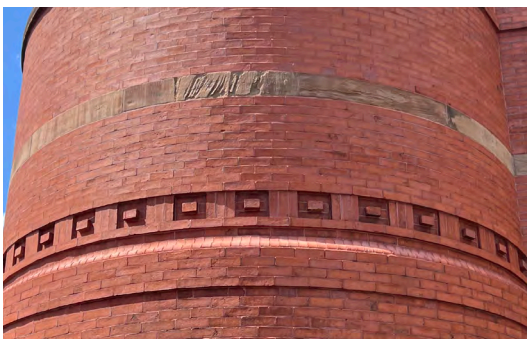
Image A-31: View of brownstone and brick banding at the turret. Note the erosion at the brownstone band.
