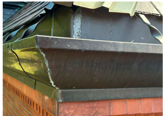
Image A-18: Typical k-style copper gutter at south west corner of the Town Hall. Note the open miter joint.
