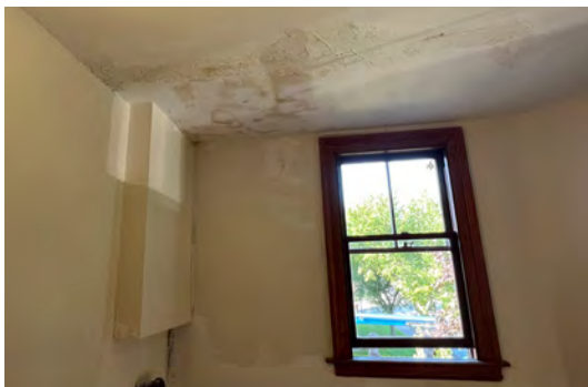
Image B-08: Interior damage at southwest stairwell caused by chronic roof leaks.
