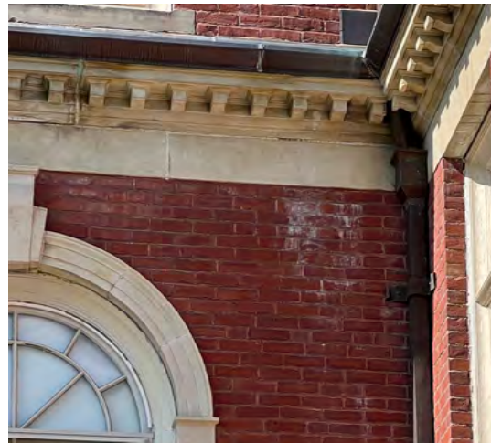
Image B-23: Staining and efflorescence at sandstone cornice and brick masonry caused by leaking gutter and downspout.
