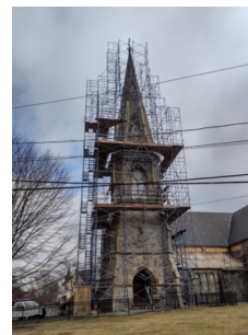
Newton Grace Episcopal Church 76 Eldredge St $1.43 million from City's CPA Also receiving funds from Mass Historical Commission Restore belfry and clock Under construction
