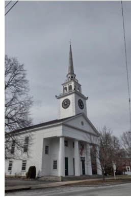
Billerica First Parish Church 7 Concord Road $52,977 Repair church steeple, weathervane and renovate clock Completed 2020
