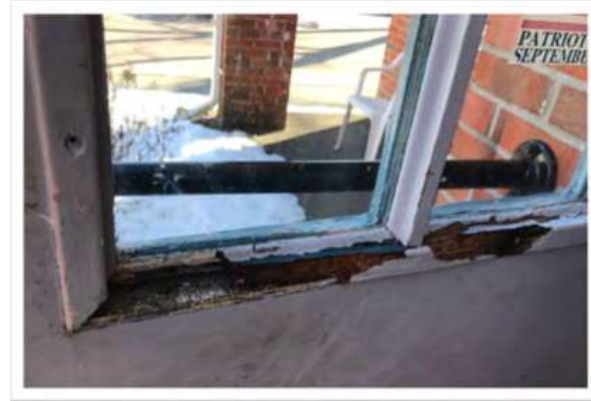
Rust and failing joint sealant
