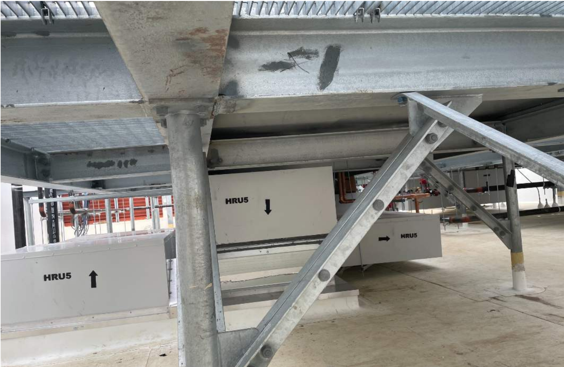
Mechanical Well Grating and Ductwork
